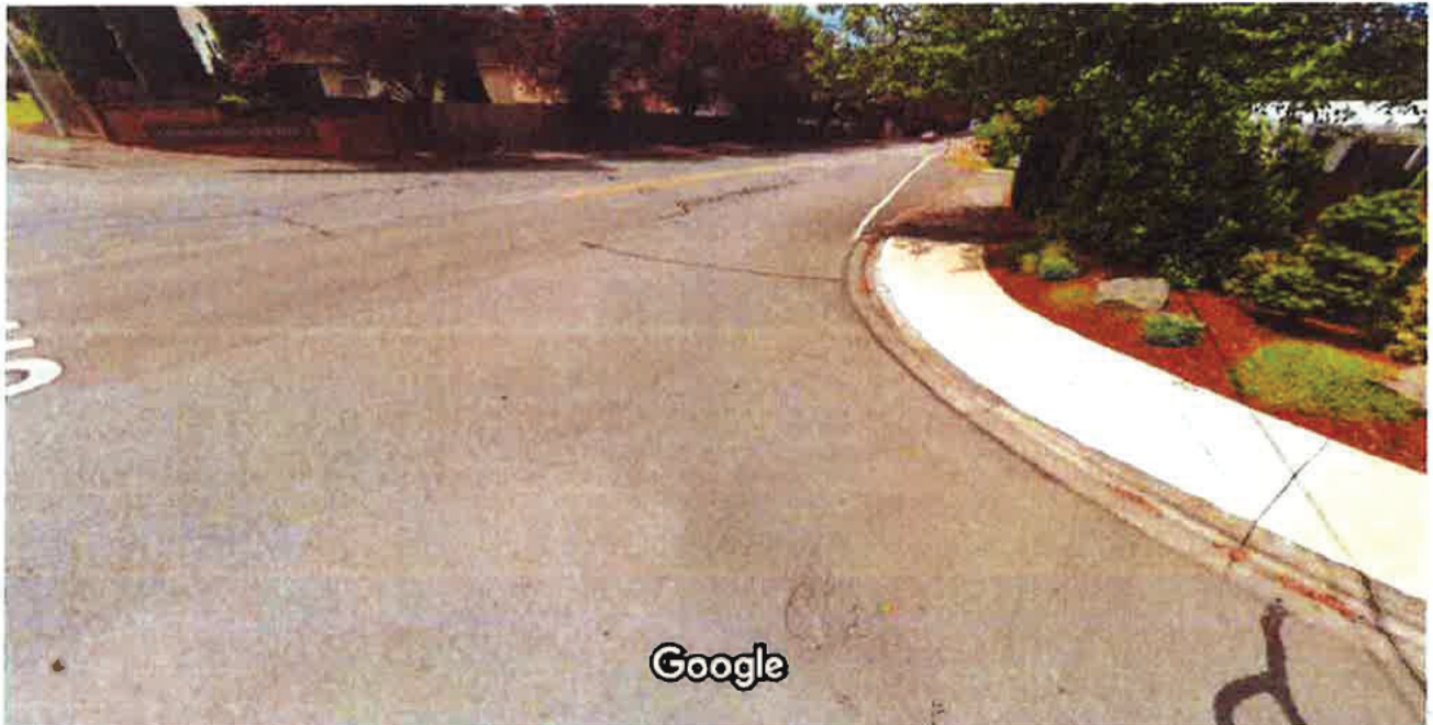
Cinnamon Hills PI (North Side) Looking West No sight distance issues, however existing ADA ramp does not meet standards No existing pedestrian ramp for crossing Sunset Blvd.
