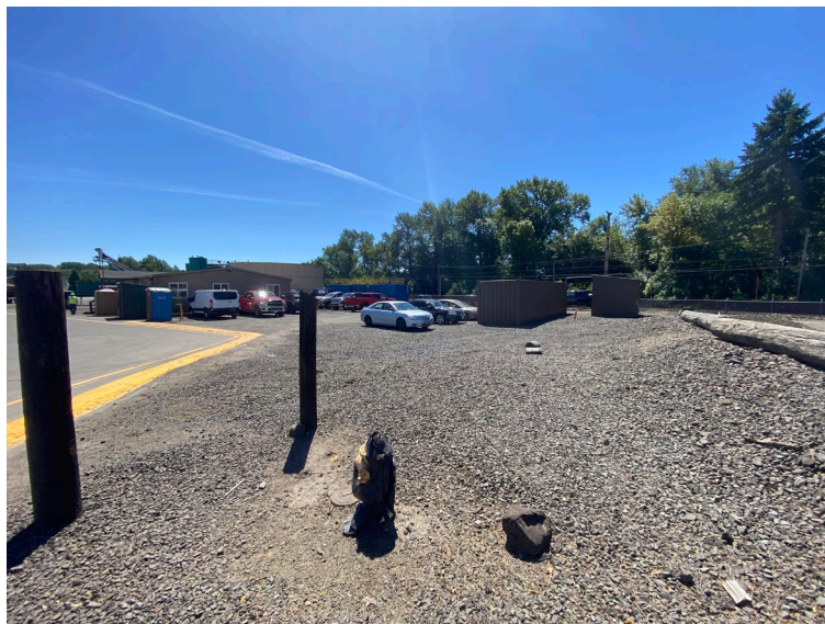
Image 1 – Fire Hydrant Repair Area
