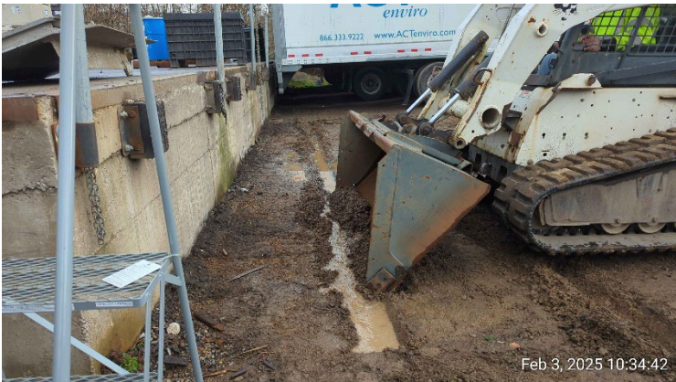
A skid steer was used to facilitate sample collection within the compacted surficial gravel.
