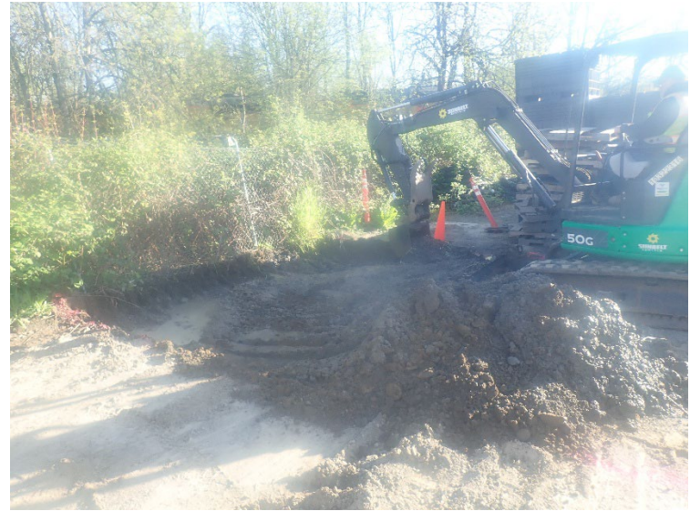
On April 18, 2025 additional soil was removed by ACT from both acid spill areas (DU01 and DU02).
