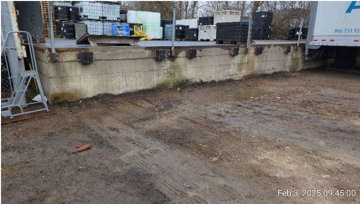
View of loading dock where the February 2024 acid spill occurred (DU01). Photo taken February 2025 during ENW's ISM sample collection.
