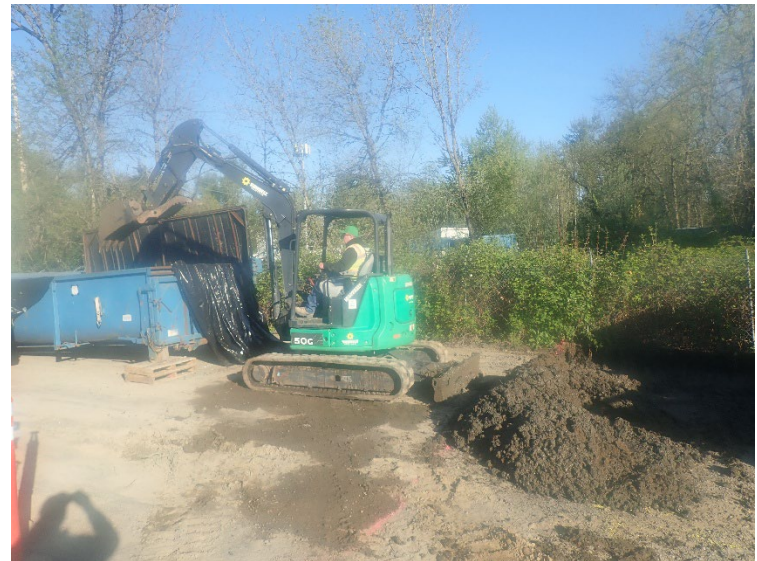
Excavated soils were placed into 10-yard drop boxes for appropriate offsite disposal coordinated by ACT.
