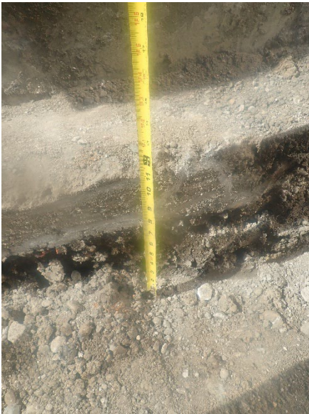
At least one foot of soil was removed from each acid spill area based on sample data collected during ENW's assessment.
