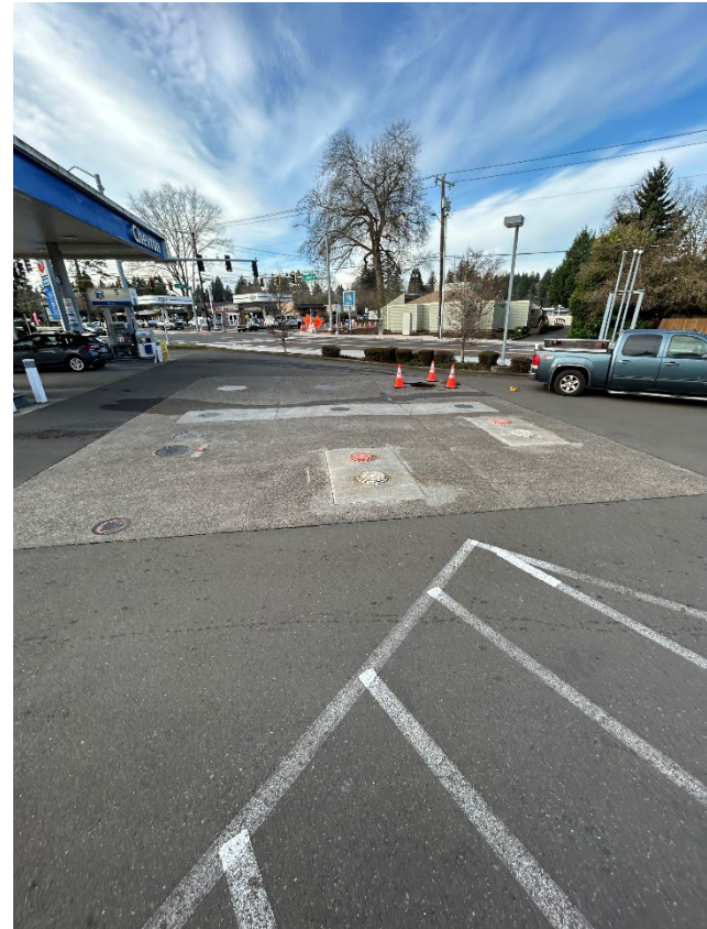
2: Tank nest looking south
