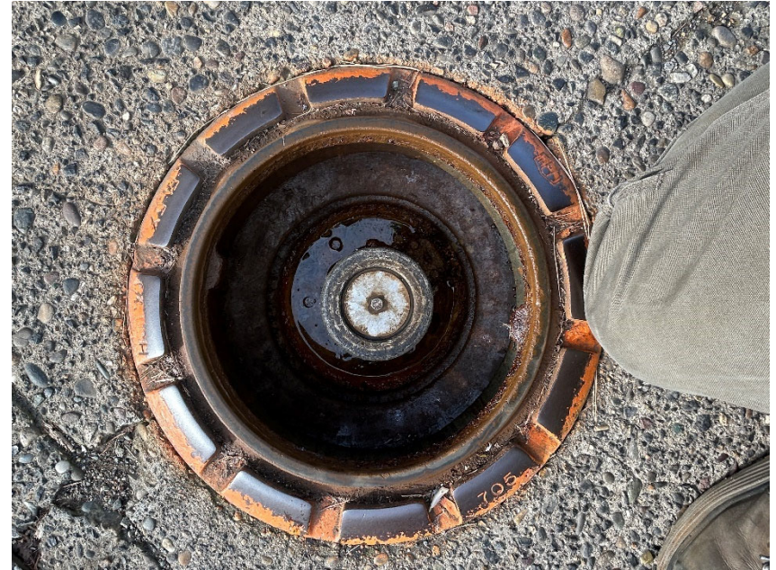
40: Regular vapor recovery #1
