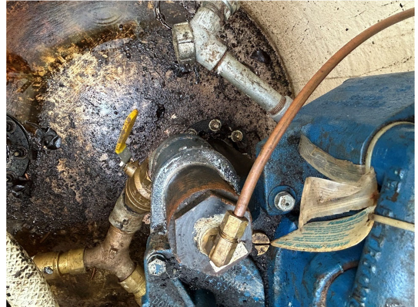
30: Regular sump #1 – leak detector
