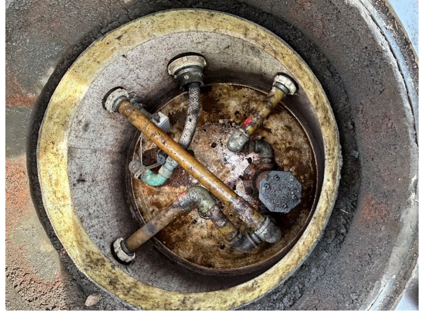
32: Regular transition sump
