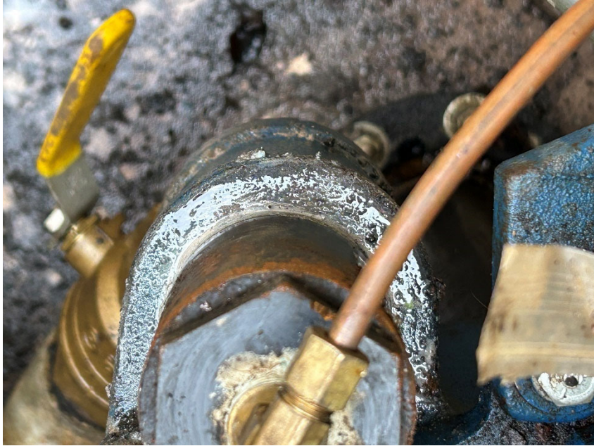
31: Regular sump #1 – leak detector, product appears to be weeping from LD.
