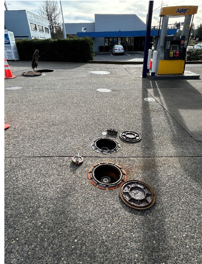
36: Regular fill and vapor recovery #2
