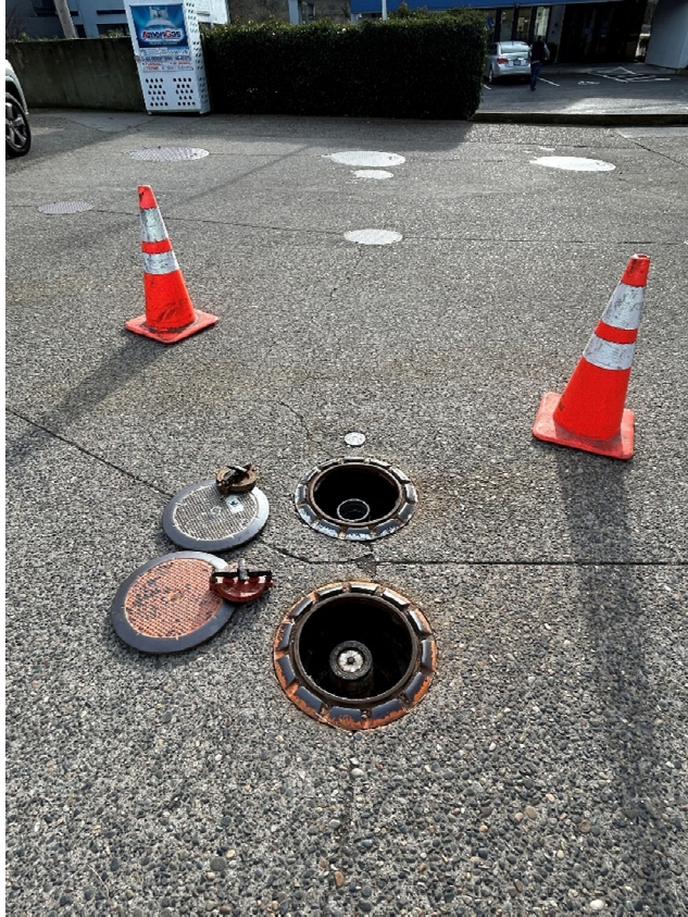
39: Regular fill and vapor recovery #1
