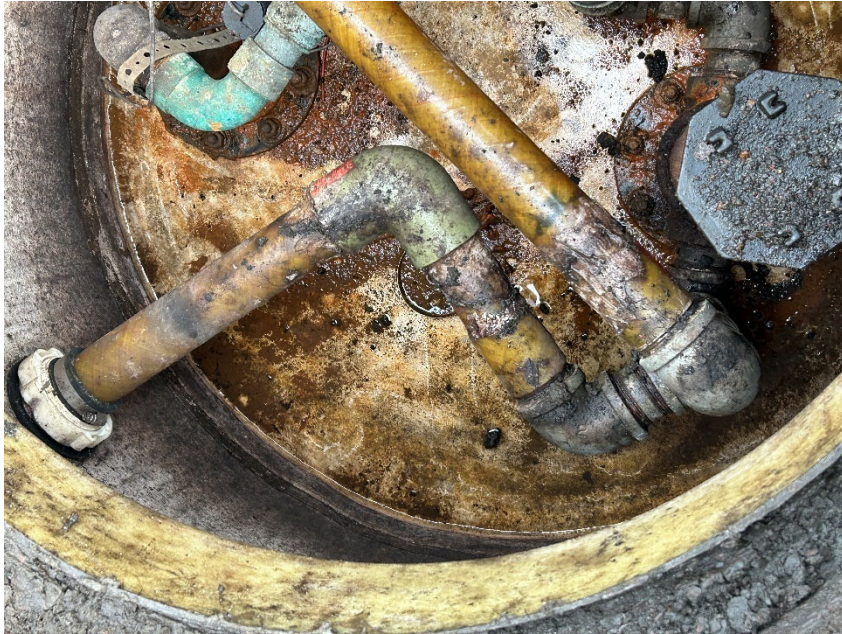
35: Regular transition sump
