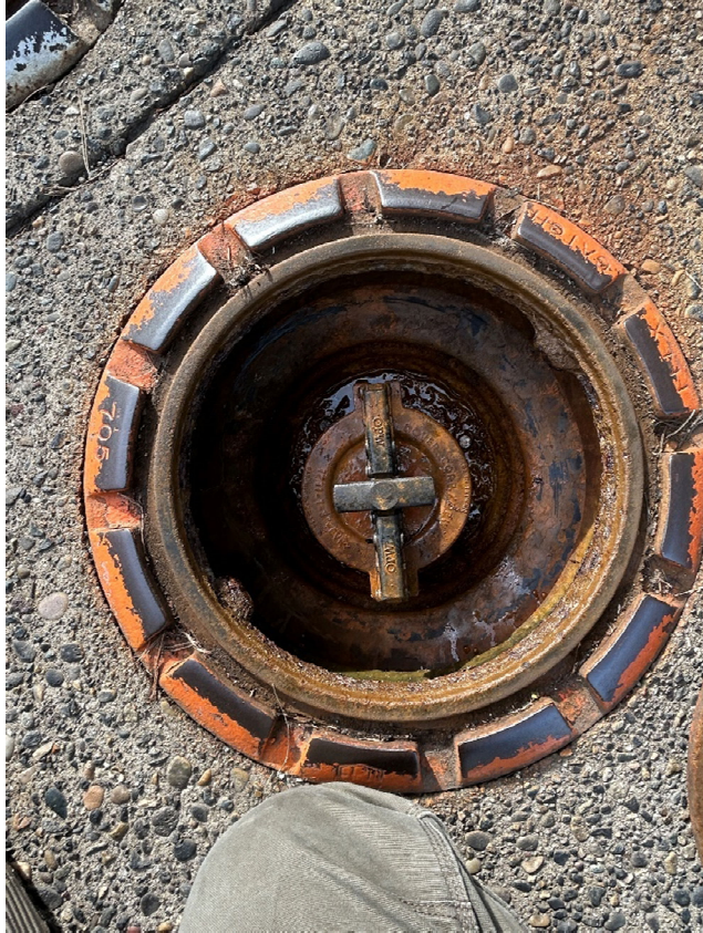
37: Regular vapor recovery #2
