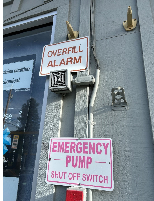
20: Overfill alarm and emergency shut off
