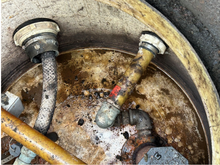
33: Regular transition sump
