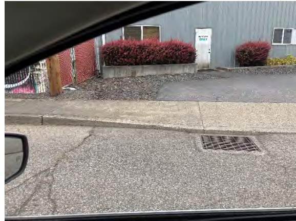
Photo #3 ANB991: Potentially receiving from 9130 N Burrage Ave – Tax Lots 2400 & 2500 (view from N Frontage Rd)
