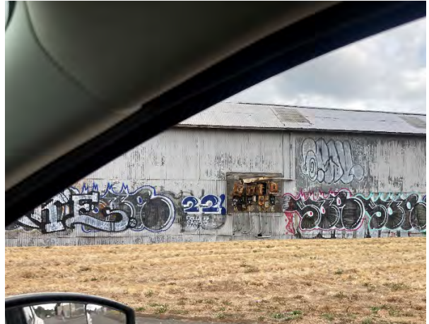
Photo #2 Dilapidated electrical panel – Just north of ANB990 (view from N Frontage Rd)
