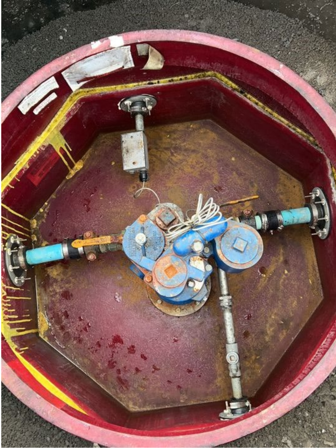
Reg 2 sump manifolded
