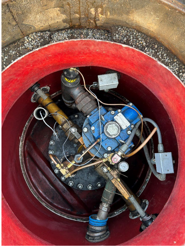
9: Diesel sump #2 manifolded using siphon breaks
