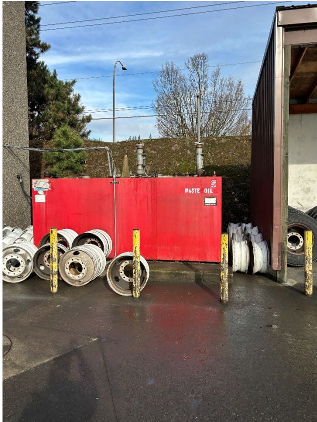
16: Above ground waste oil tank
