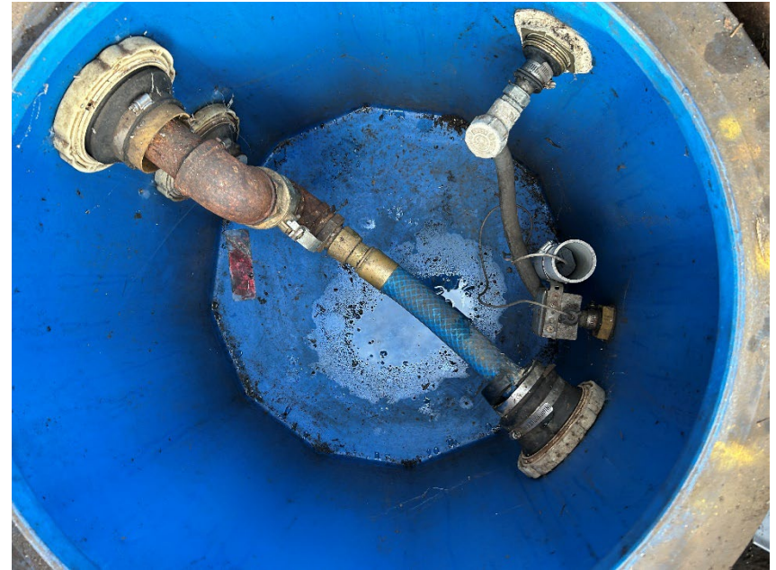
17: Waste oil transition sump
