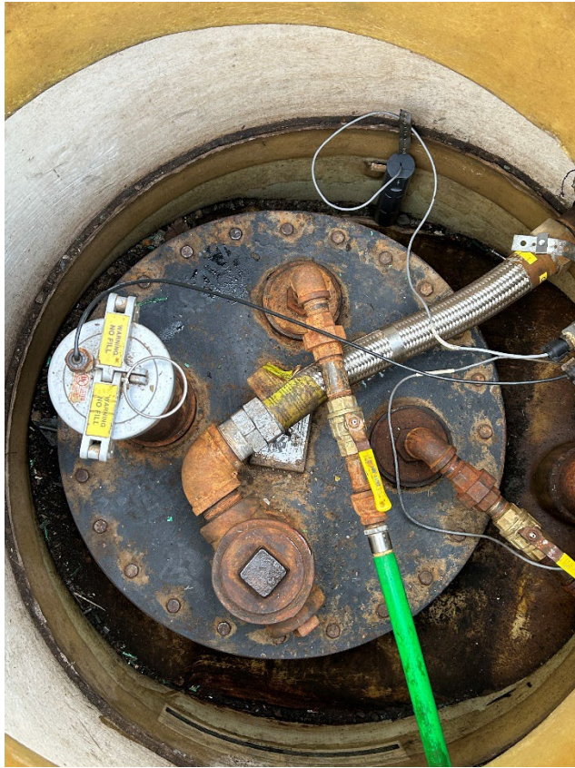
28: Sump for Egen tank
