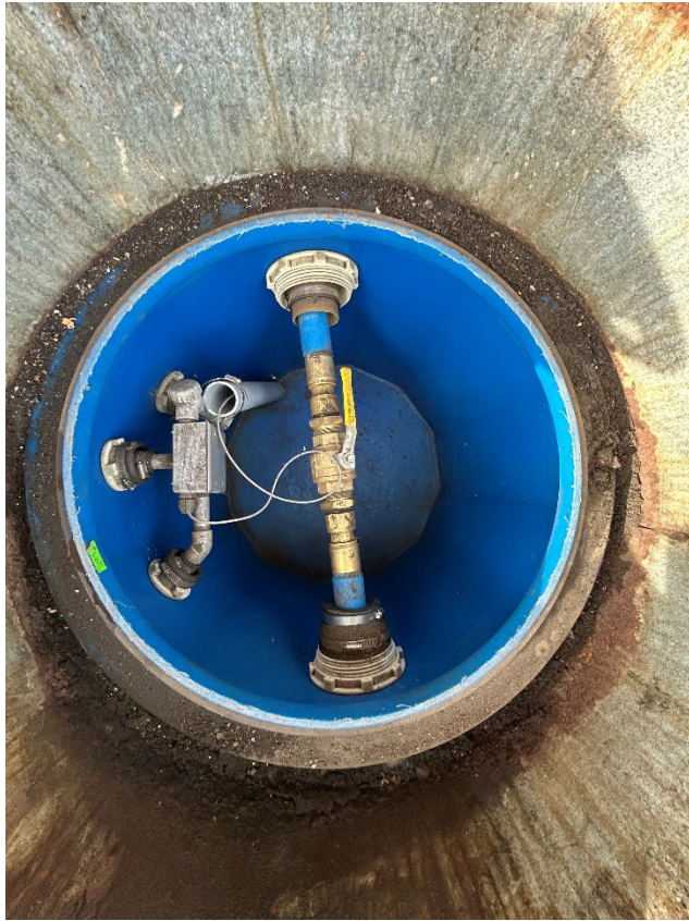
12: Transition sump to dispensers
