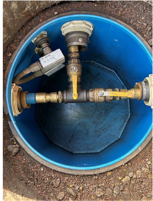
13: Transition sump to dispensers 4,5 and 6
