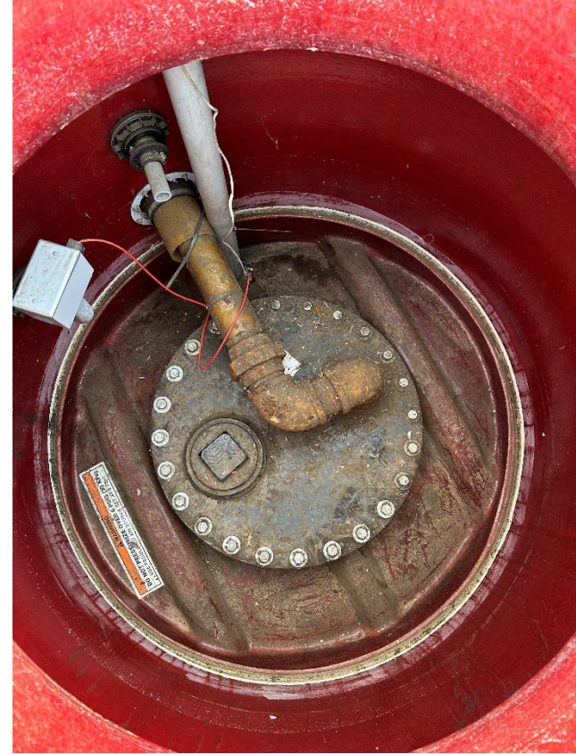
10: Diesel sump #3 manifolded
