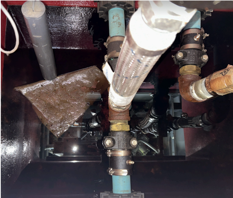
UDC ¾ - Leaking Diesel Meter – Raised
