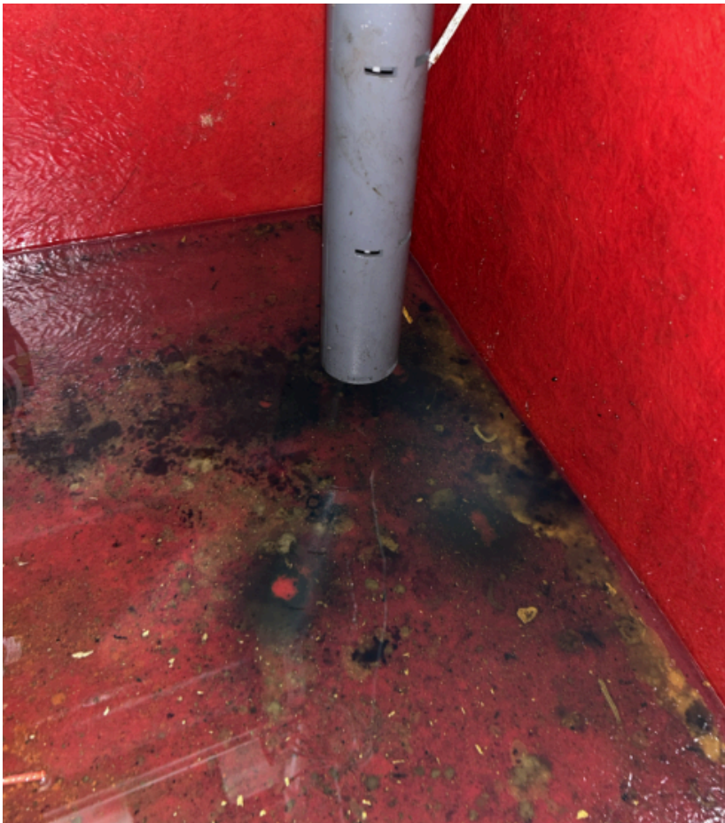
UDC 11/12 – Leaking Meter – Raised Sensor
