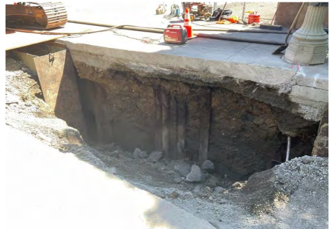
Photo 4: Contamination in Bursting Pit - NW 9th Ave and Johnson
