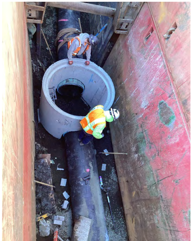
Photo 14: HDPE Storm Pipe and Maintenance Hole - NW 9th Ave at Kearney
