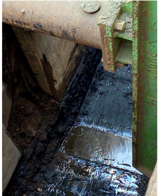
Photo 8: Petroleum Sheen on Groundwater - NW 9th Ave between Lovejoy/Kearney
