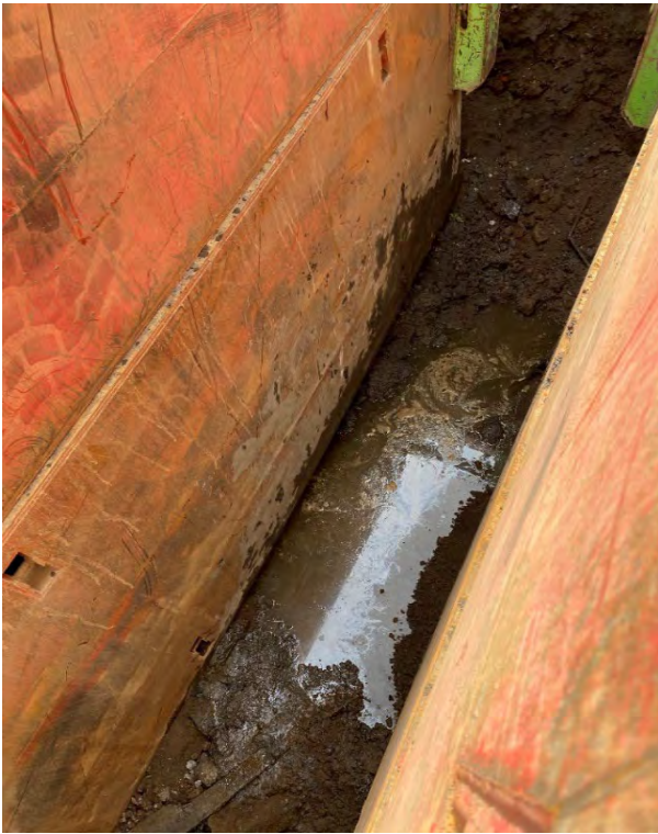
Photo 11: Petroleum Sheen on Groundwater - NW 9th Ave between Kearney/Johnson
