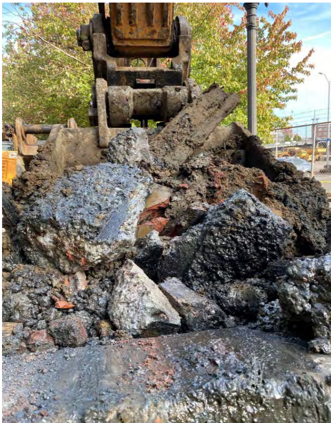
Photo 9: Petroleum Saturated Debris - NW 9th Ave and Kearney
