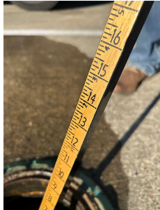
8: 14" of diesel in the tank
