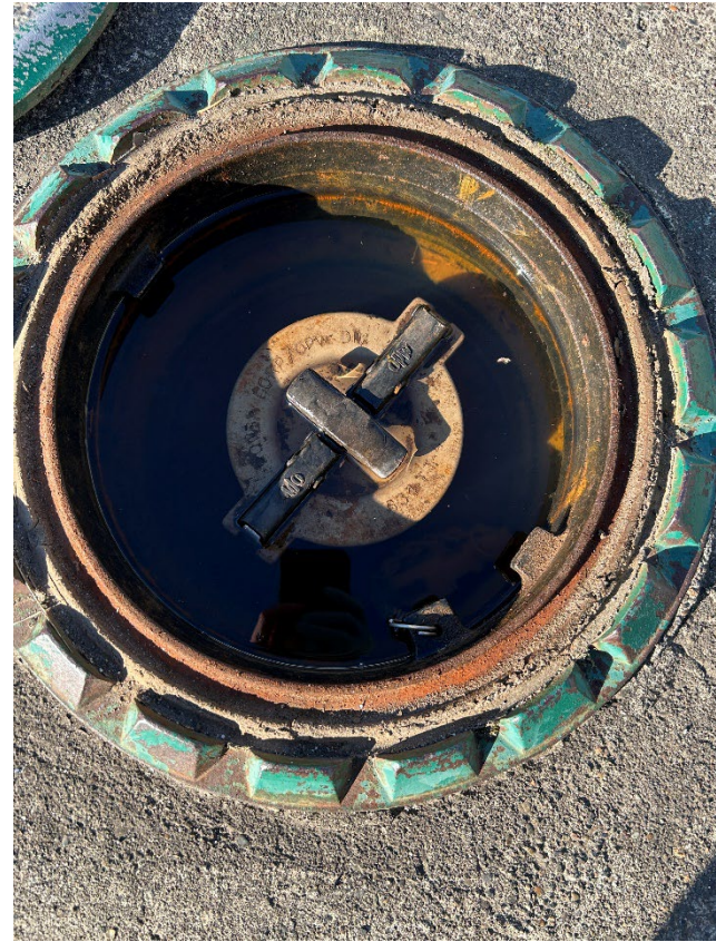
6: Diesel spill bucket with water present
