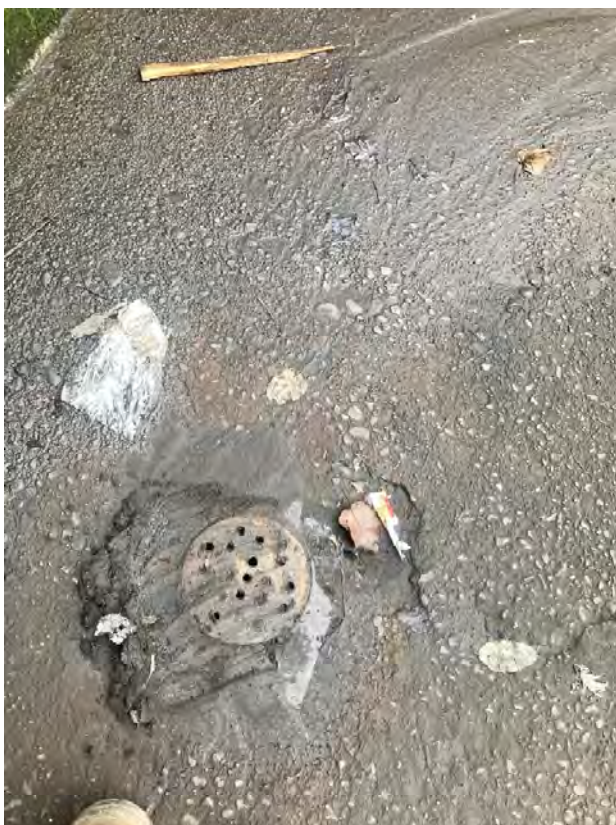
Inlet at loading dock on east side of property with unknown discharge location. 1/29/21; K. Balogh
