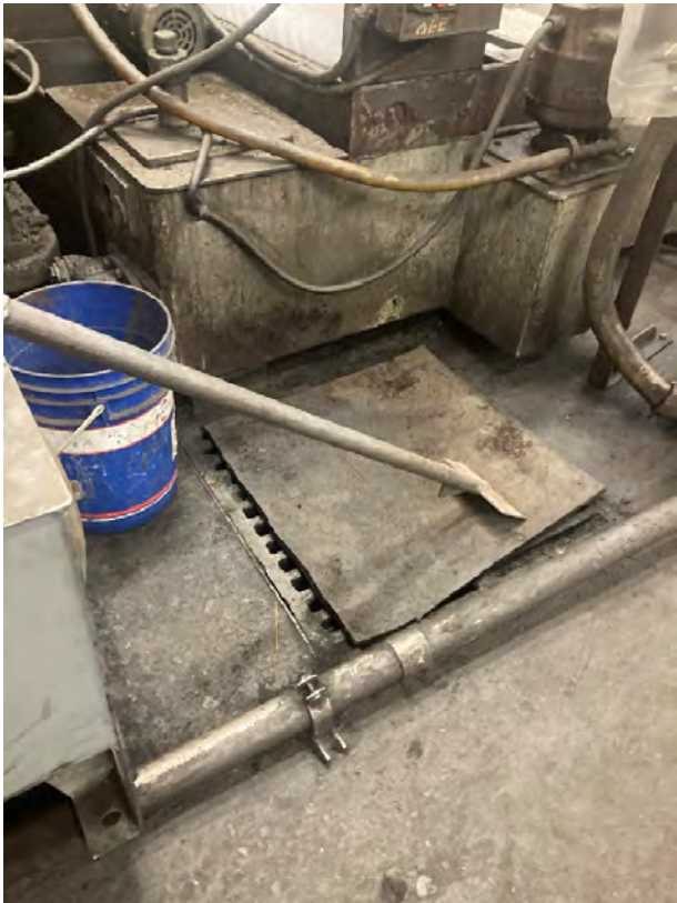
Interior floor drain under surface grinder, 11/23/20; K. Balogh
