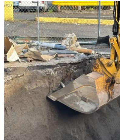
Photo #6 Sampling soil under kerosene product piping.
