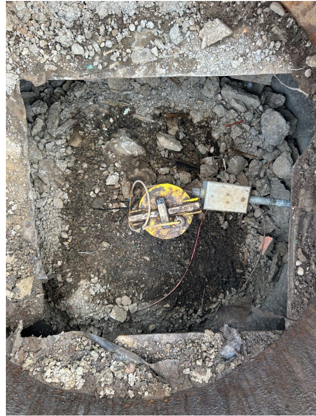
12: Diesel tank gauge probe
