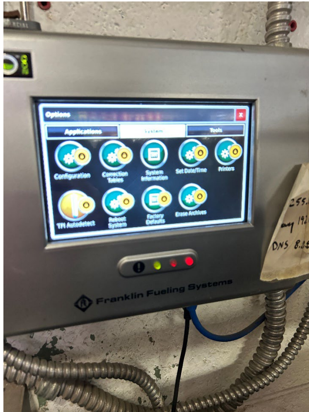
5: No access to set up report
