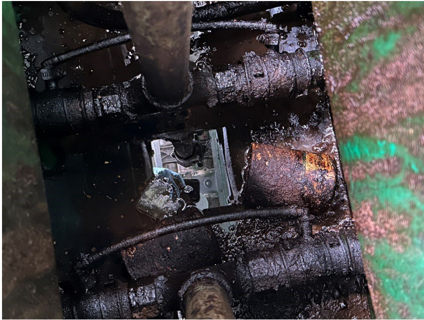
21: UDC #7/8 with filter oil in bottom
