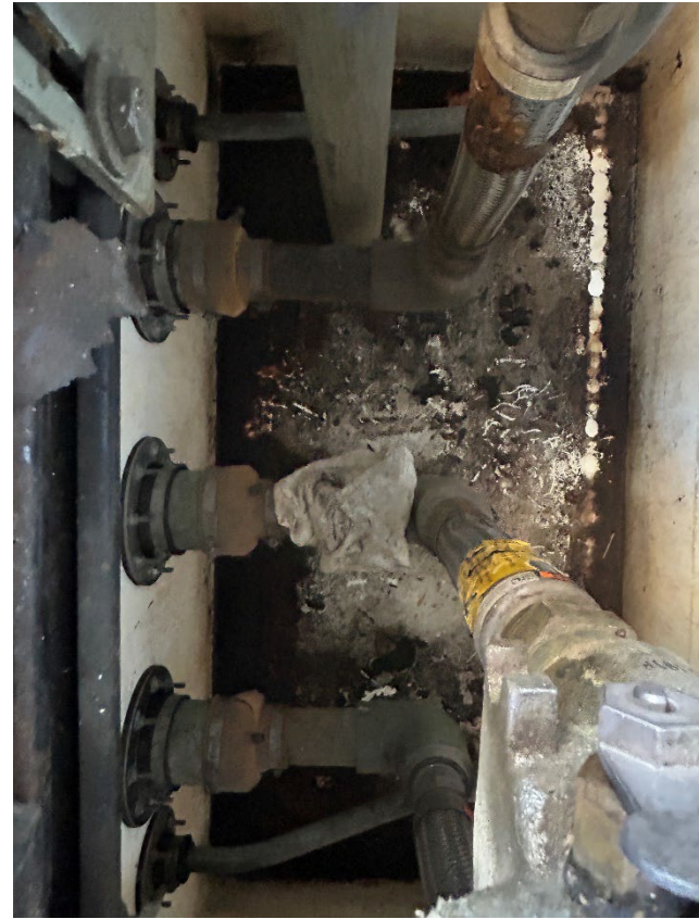
18: UDC #1/2 all boots broken
