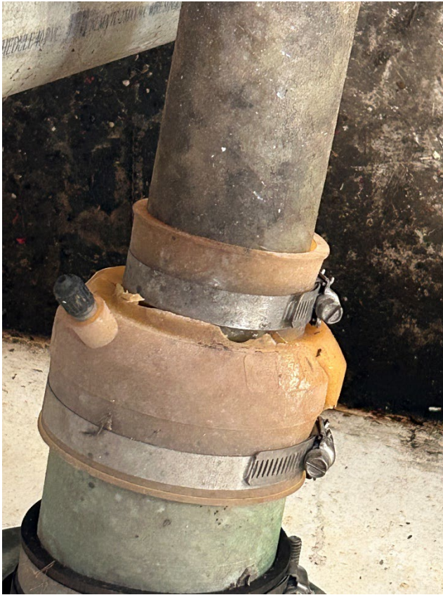
17: Broken boot in UDC #3/4
