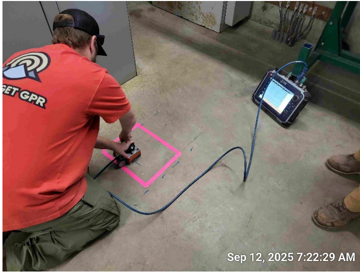
Ground-penetrating radar was used to help site sub-slab sample locations within the lowest level of the RJH building.
