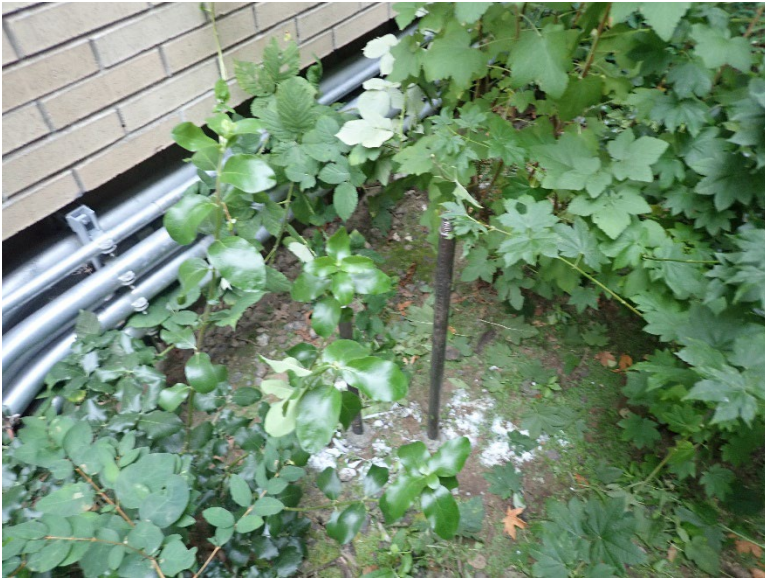
At each soil gas sample location, temporary soil gas probes were installed to collect samples at both 5- and 10-foot depth intervals.
