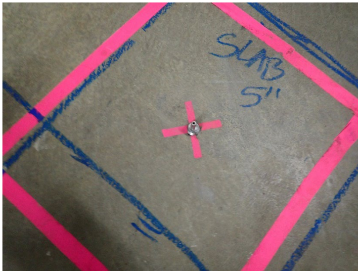
View of vapor pin installed at location SUB01 within the RJH building.
