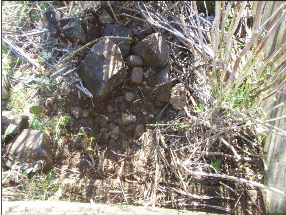
Photo G. Plot 1 location after digging amidst the cobble, rubble, and debris.
