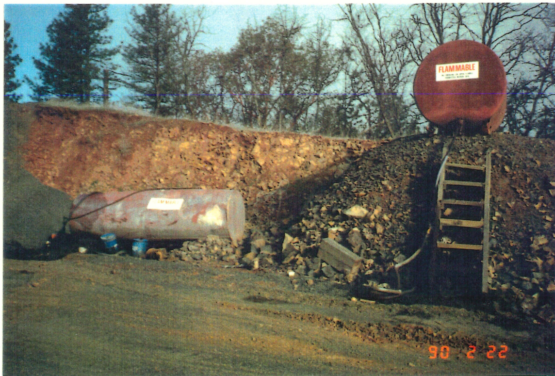
Figure 19: Above ground storage tanks at the 140 Quarry site. The surface soil around the distribution lines is heavily stained.
