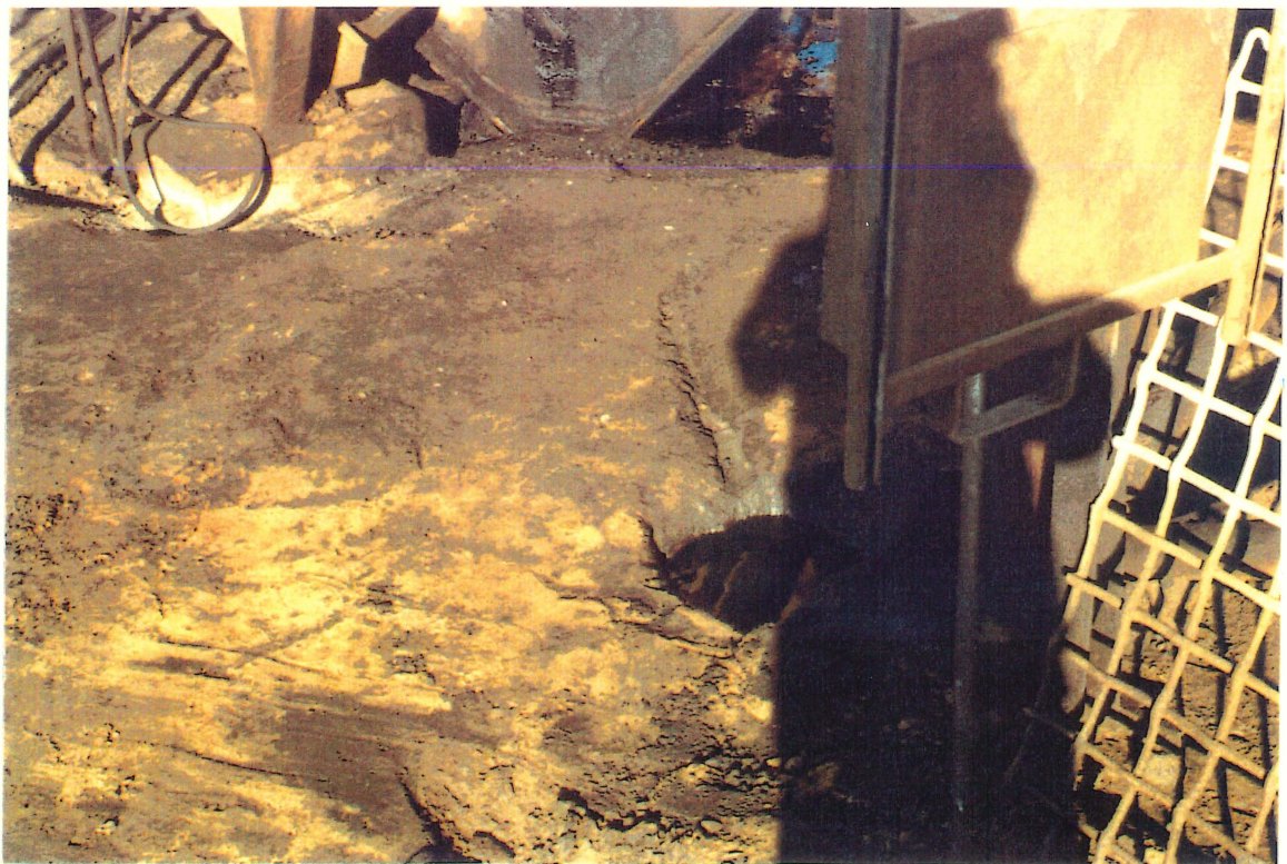
Figure 13: Hole, excavated and filled by Villas site personnel, containing a diesel/water mixture.
