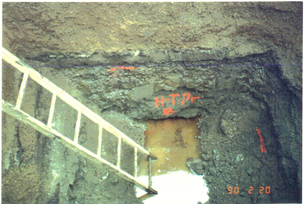
Figure 8: Hamrick site test pit H-TP-8. Petroleum-rich water is leaking out of the gravelly layer at the upper paint line. The paint lines are soil sample points. Groundwater, intercepted at 8.0 feet below grade, contains heavy oil and a lighter petroleum product.
