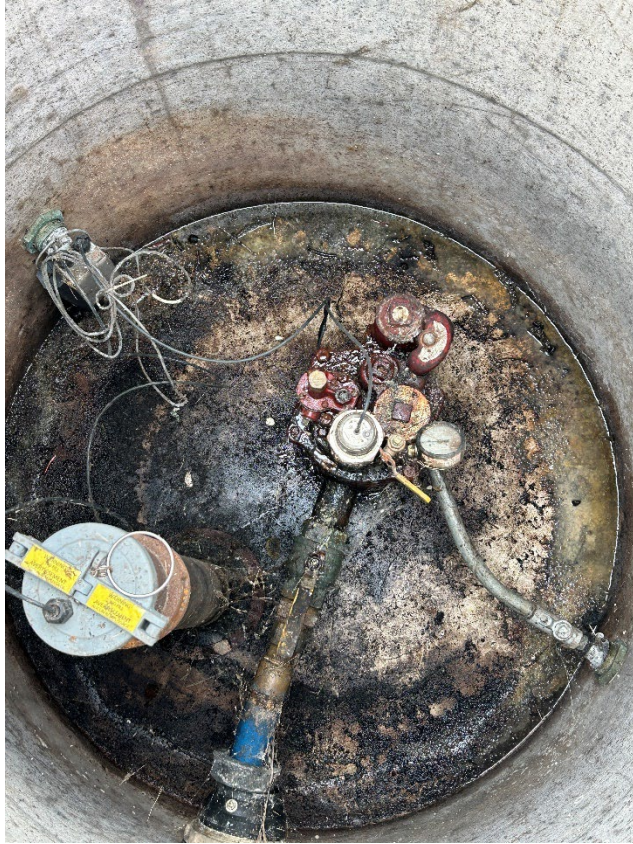
7: Sump for UST #2 gasoline
