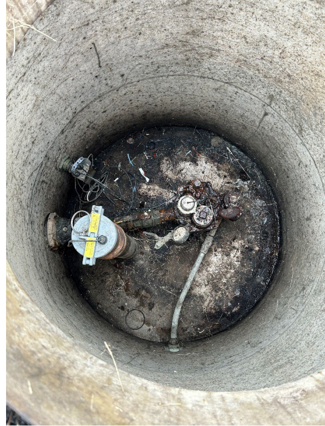
8: Sump for UST #1 Diesel
