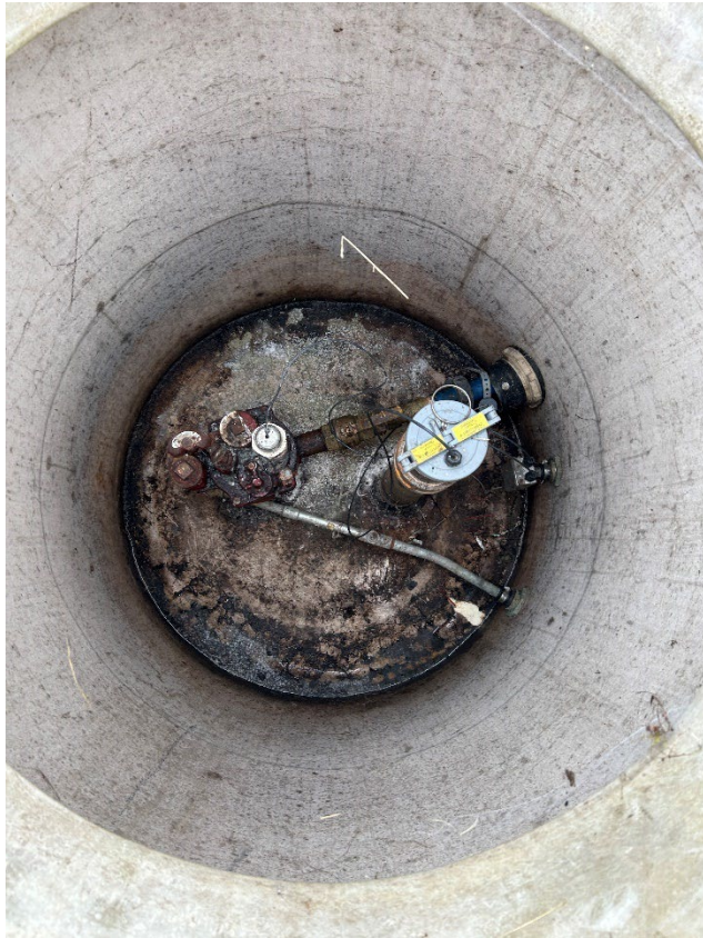
11: Sump for UST #3 Diesel
