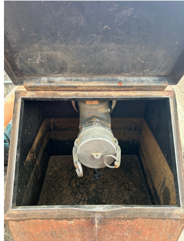
4: Above ground fill for gasoline
