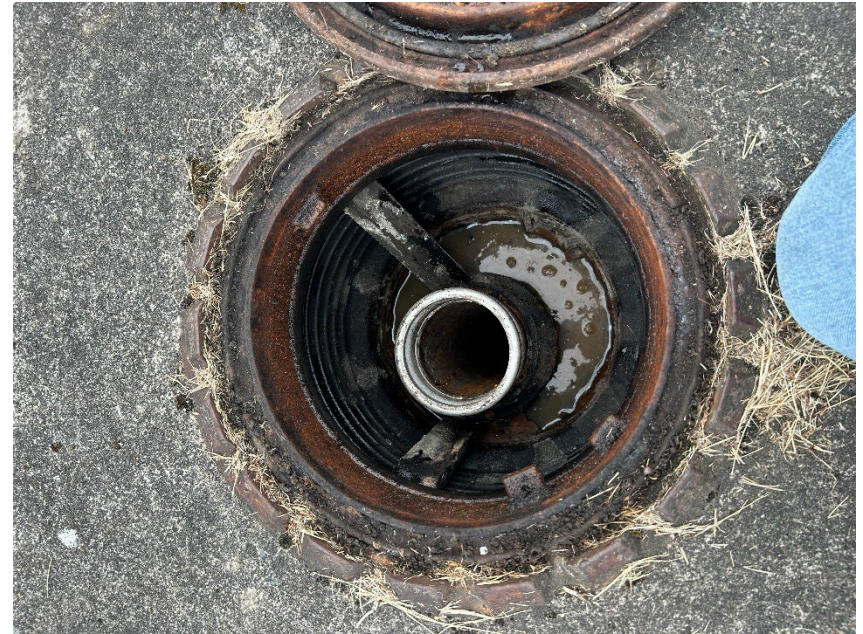
10: Unused fill ports on top of berm tanks area
