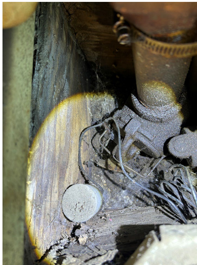
8: Spike anode below Diesel Disp
