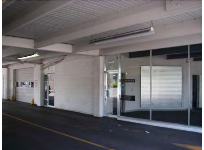
10. 4403 Commercial St. SE: View of the breeze way/canopy area and south side of the Main Building. View also shows fluorescent lighting.
