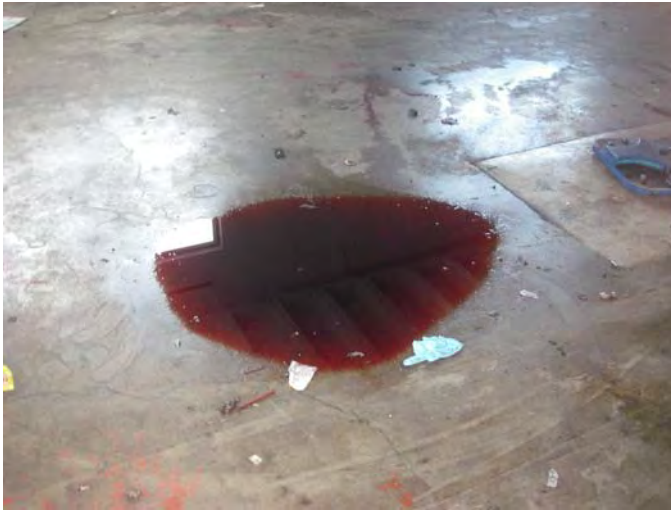
31. 4516 Sunnyside Rd SE: Representative view of freestanding oil observed on concrete surface and adjacent to hydraulic lifts in the former "Firehouse" building.
