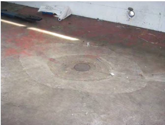
33. 4516 Sunnyside Rd SE: View of the decommissioned floor drain located in the former "Firehouse" building.
