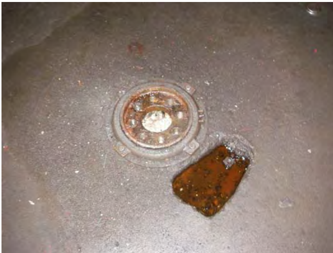
17. 4403 Commercial St. SE: Representative view of a below-ground hydraulic hoist and freestanding oil on asphalt-paved surface in the Main Building service area/garage.
