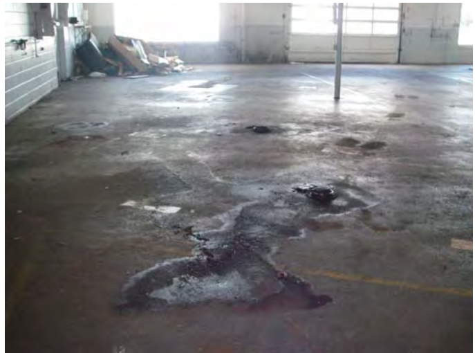
18. 4403 Commercial St. SE: Interior view of the Main Building service area/garage showing below-ground hydraulic hoists, freestanding oil and surface staining, and the non-hazardous trash/debris pile in the distance.
