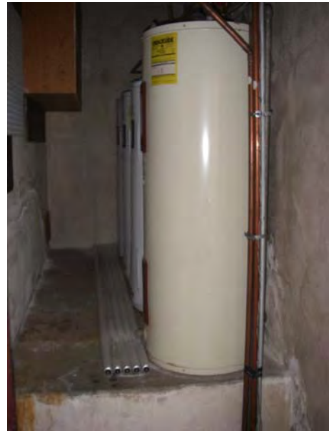
34. 4516 Sunnyside Rd SE: Room with hot water heaters on the second floor of the former "Firehouse" building.
