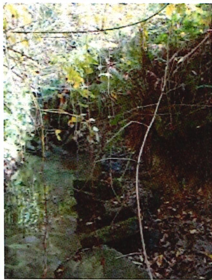
West Bank Chehalem Creek Streambank Erosion
