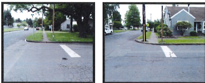
FIGURE 1 CURB RAMP NEEDED
