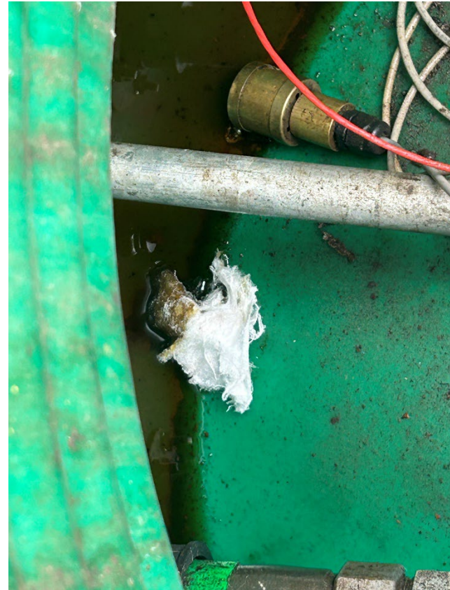
10: Product present in diesel sump #1
