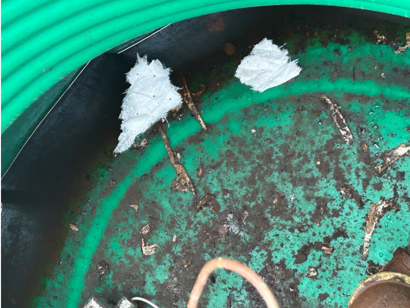
13: Small amount of water in diesel sump #2
