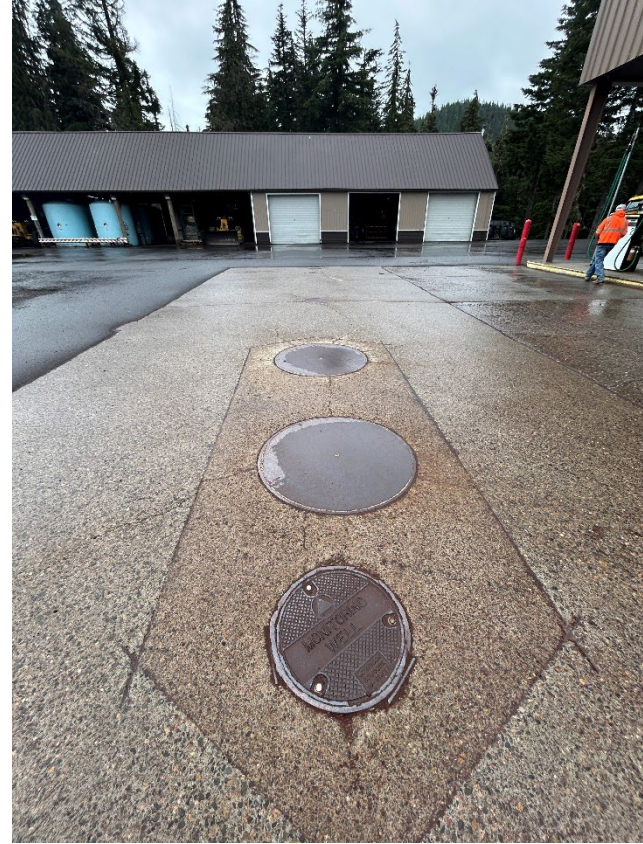
2: Tank nest looking south
