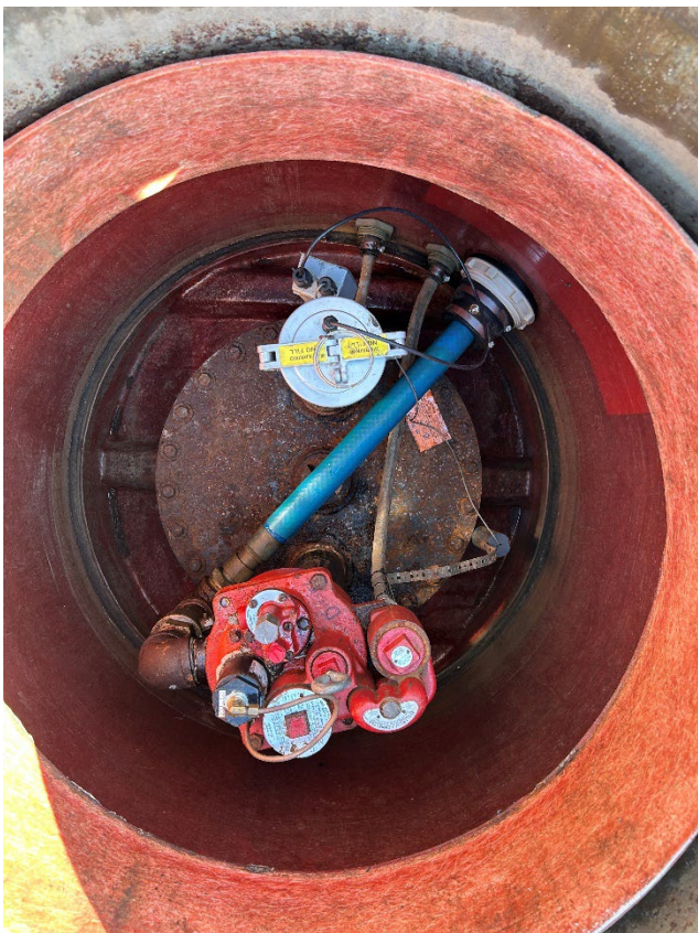
5: Diesel tank-top sump
