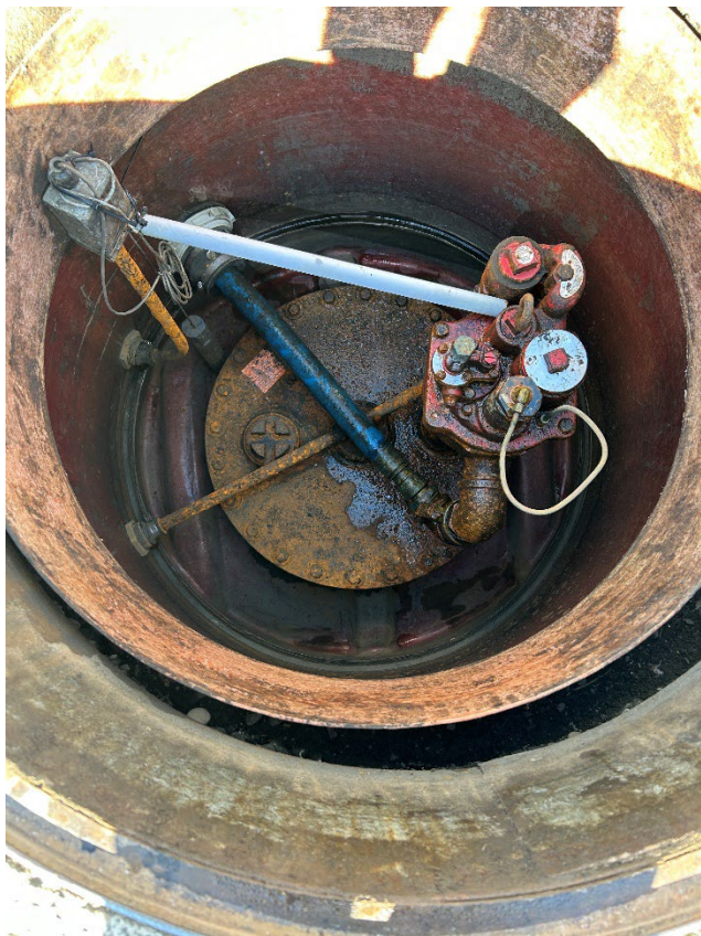
7: Regular tank-top sump
