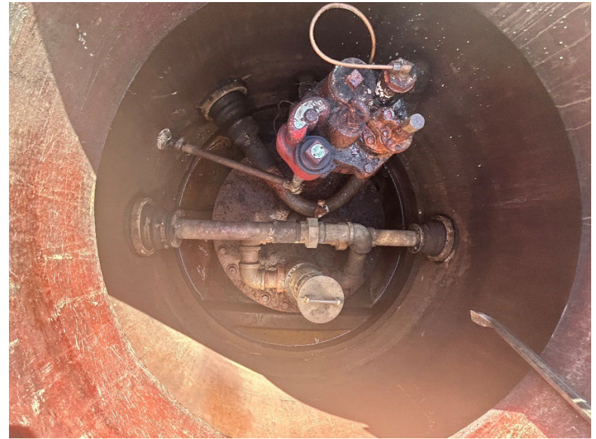
10: Regular sump with confirmed product in bottom
