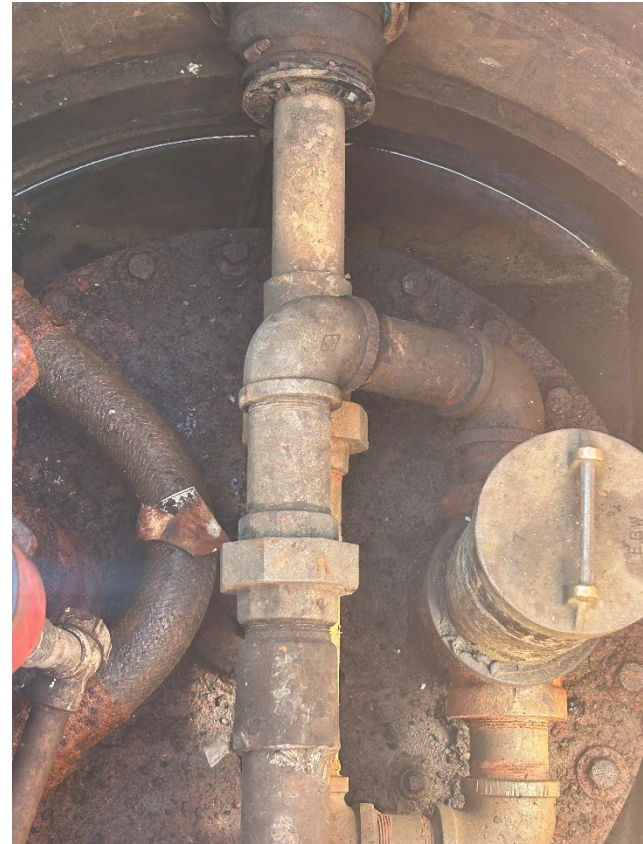
12: 2" Fiber plastic piping in regular sump
