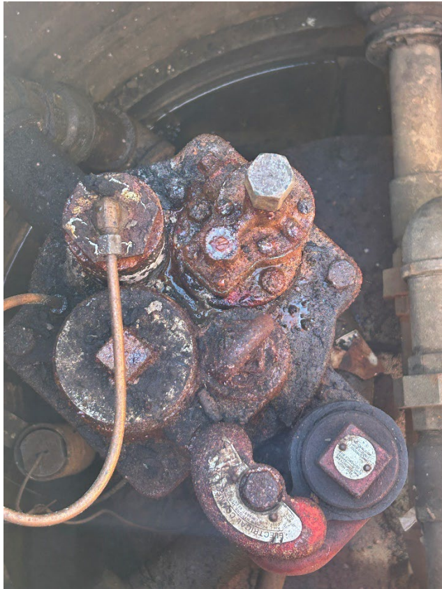
13: Red Jacket turbine in regular sump
