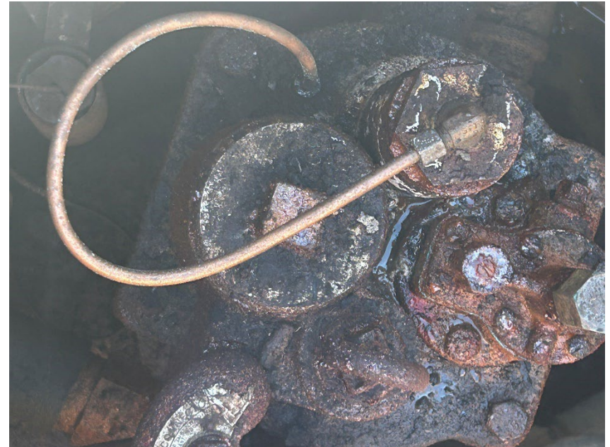
14: Top of red jacket turbine in regular sump
