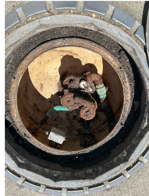
6: Diesel TT Sump
