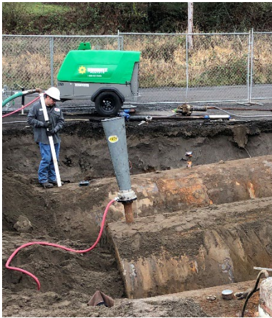
Photo #3 Ventilation of USTs
