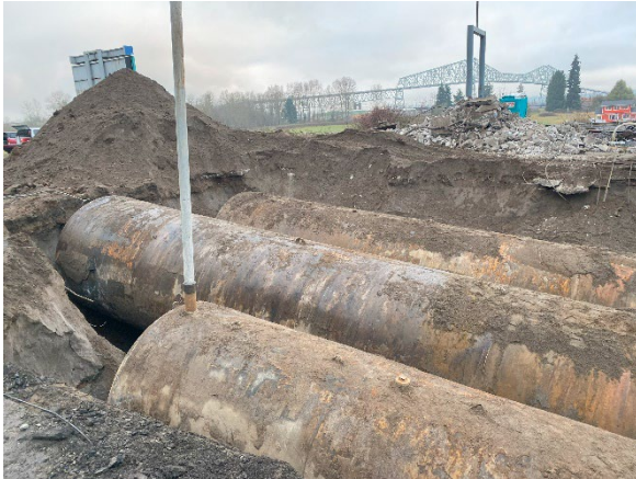
Photo #1 Three USTs, looking southeast to northwest
