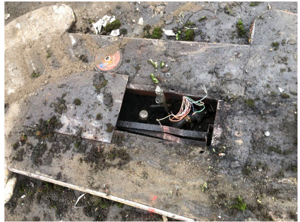
Photo #4 Dispenser locations after dispenser removal, prior to sump removal from ground
