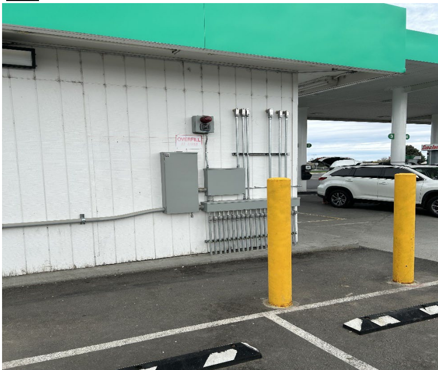
View of Overfill Alarm
