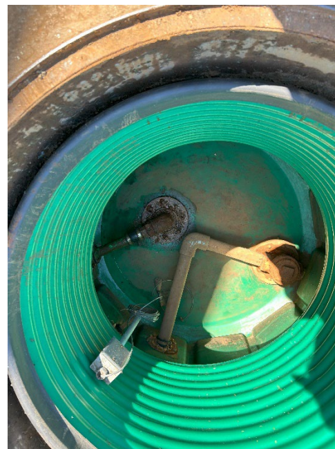
4: Diesel Manifold Sump
