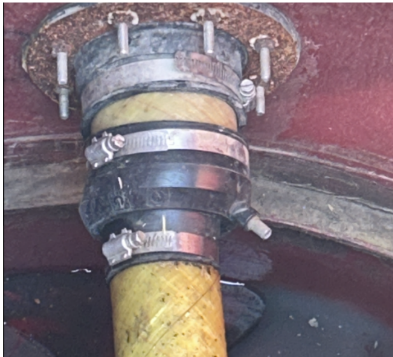
Tight boots and Shrader valve still installed.
