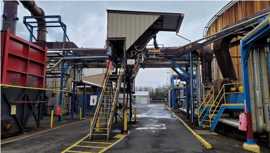
Picture 3. Typical view of truck loading rack.
