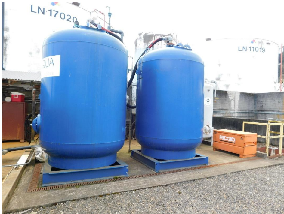
Picture 12. Unanchored water tanks at Area 02.
