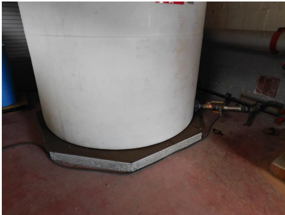
Picture 10. Unanchored foam fire tank at Area 02.
