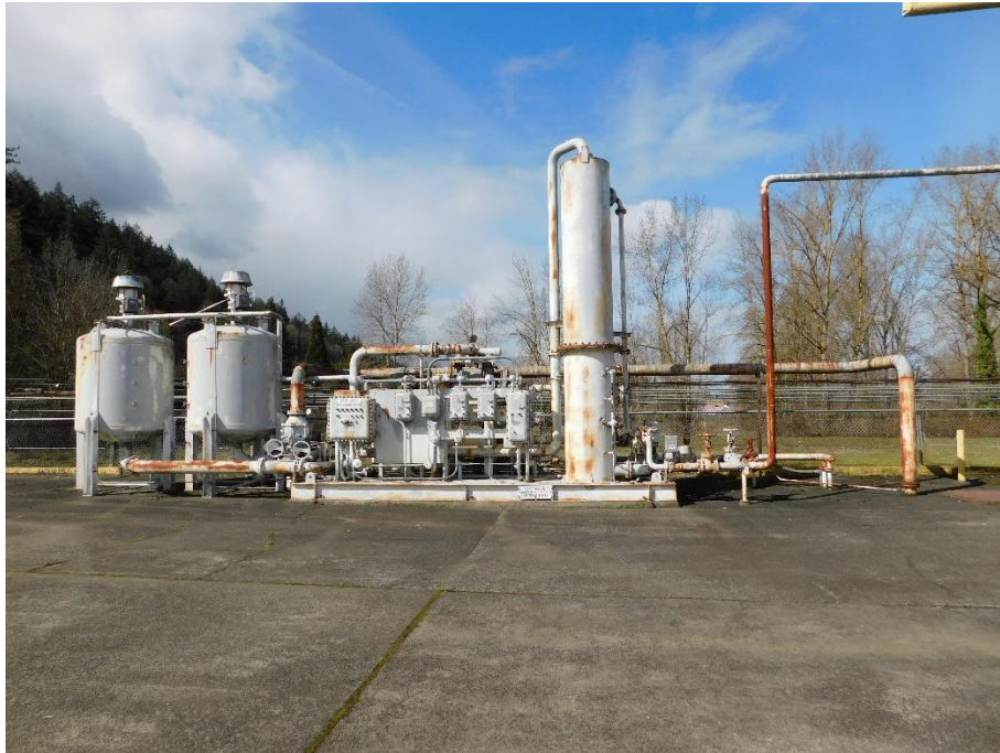
Picture 3. Typical out-of-service ancillary equipment at Area 01.
