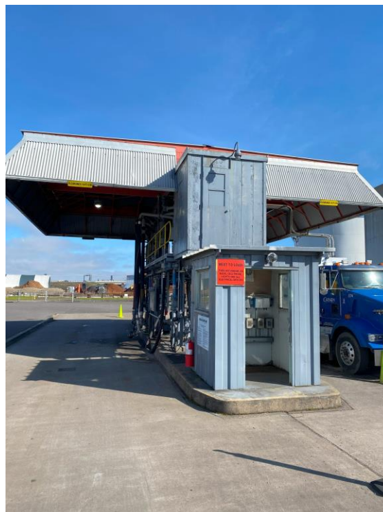
Picture 2. View of typical truck loading rack.
