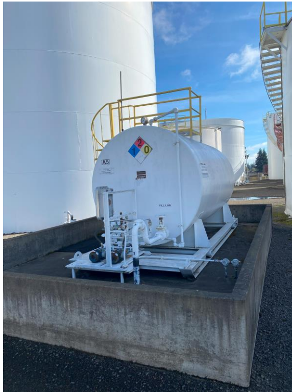
Picture 7. Typical view of unanchored additive tank.
