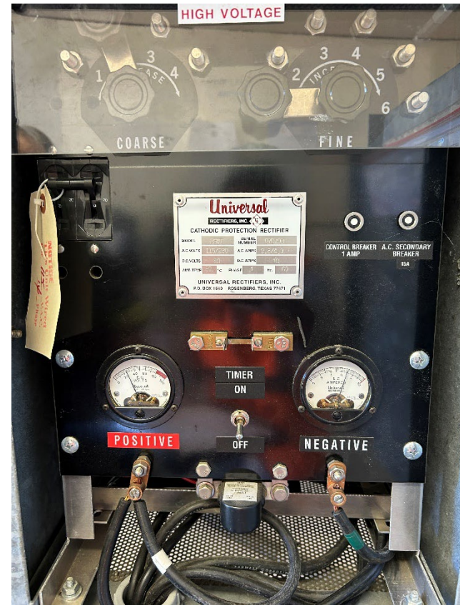
4: Impressed current rectifier
