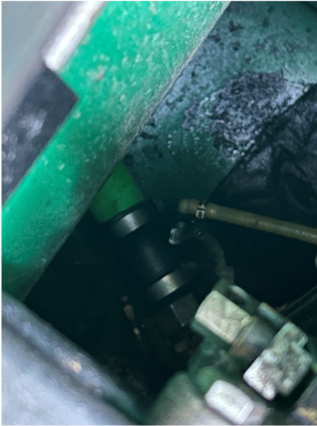
17: East Satellite diesel UDC
