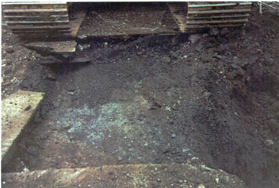
Photograph # 3: Contaminated soil beneath drainage grill.
