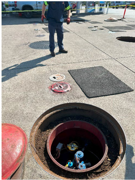
Figure 8 Chevron Regular Sump
