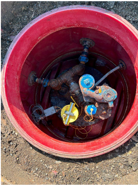
Figure 6 Chevron Regular Sump
