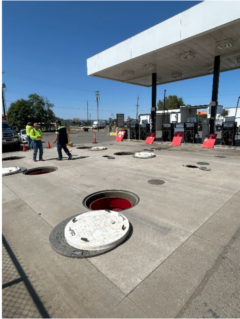
1: Tank Nest and Service Island
