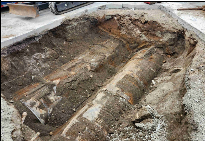
Photo #3: Exposed USTs
