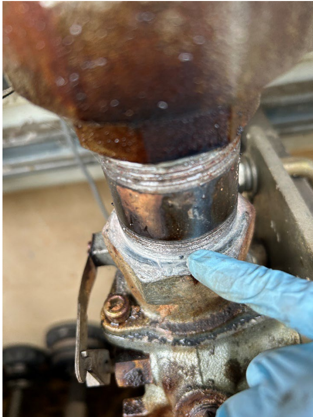
27: Weeping point on regular line in UDC #5/6
