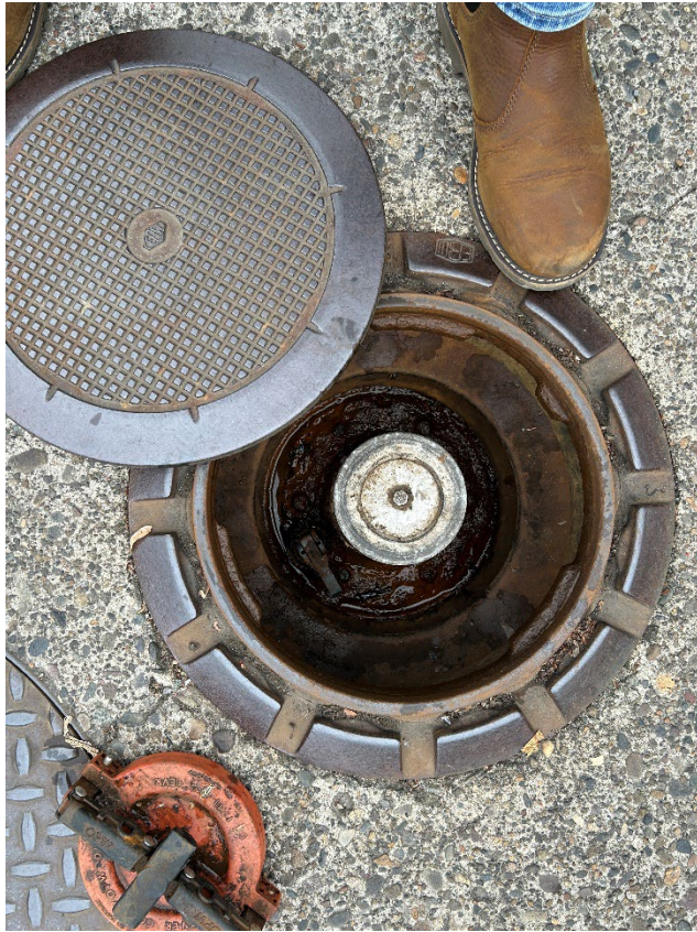
9: Old poppet valve – not in use
