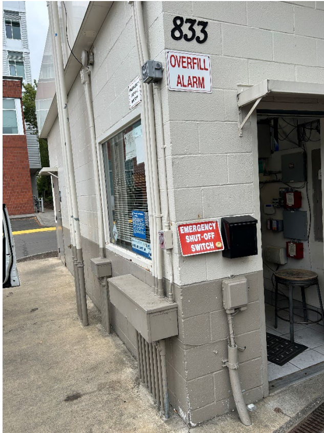
3: Overfill alarm and emergency shut-off
