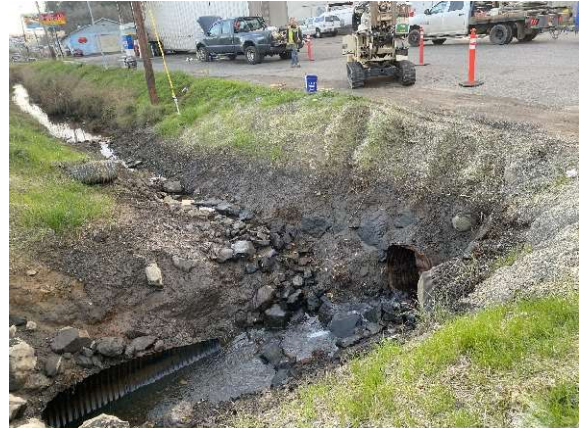
Photo #8 12/1/21: Minimal flow from drainage ditch at low tide with deeper water in the drainage ditch south of the telephone pole.
