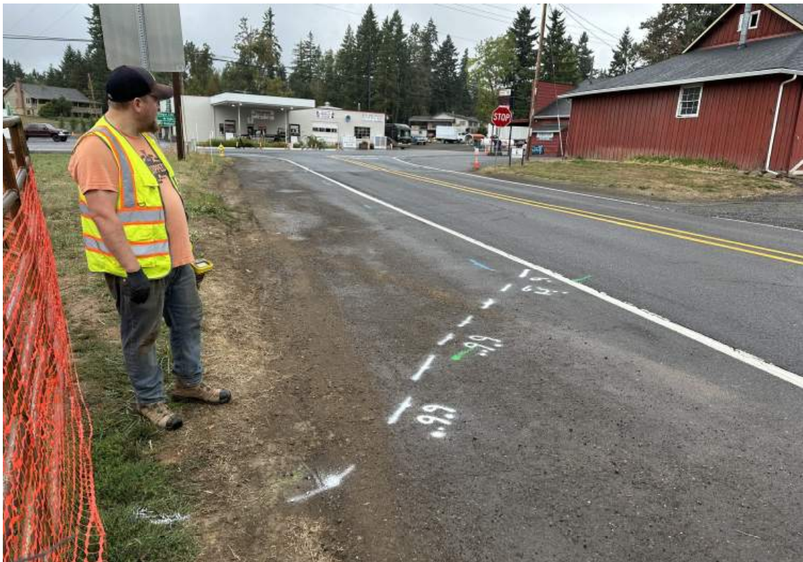
VIEW OF THE APPROXIMATE DRAIN LINE DURING UTILITY LOCATING ACTIVITIES AT THE SUBJECT PROPERTY. THE DRAIN LINE ORIGINATES AT THE REDLAND STORE.
