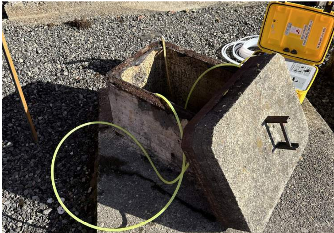
VIEW OF GREEN DYE OBSERVED IN THE REDLAND STORE FORMER UIC IMMEDIATELY FOLLOWING INSERTION OF DYE INTO THE REDLAND STORE TOILET.
