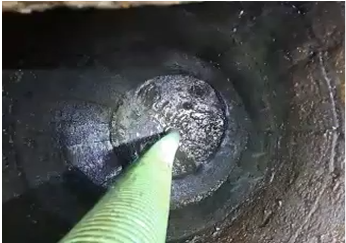
VIEW OF THE CONTENTS OF THE REDLAND STORE'S FORMER UIC DURING PUMPING ACTIVITIES.
