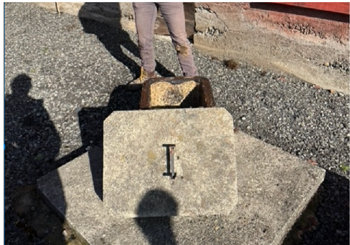
THE REDLAND STORE'S FORMER UIC MONUMENT. PHOTO TAKEN PRIOR TO REMOVAL OF A LIMITED VOLUME OF LIQUID/SLUDGE VIA SEWAGE PUMP TRUCK.
