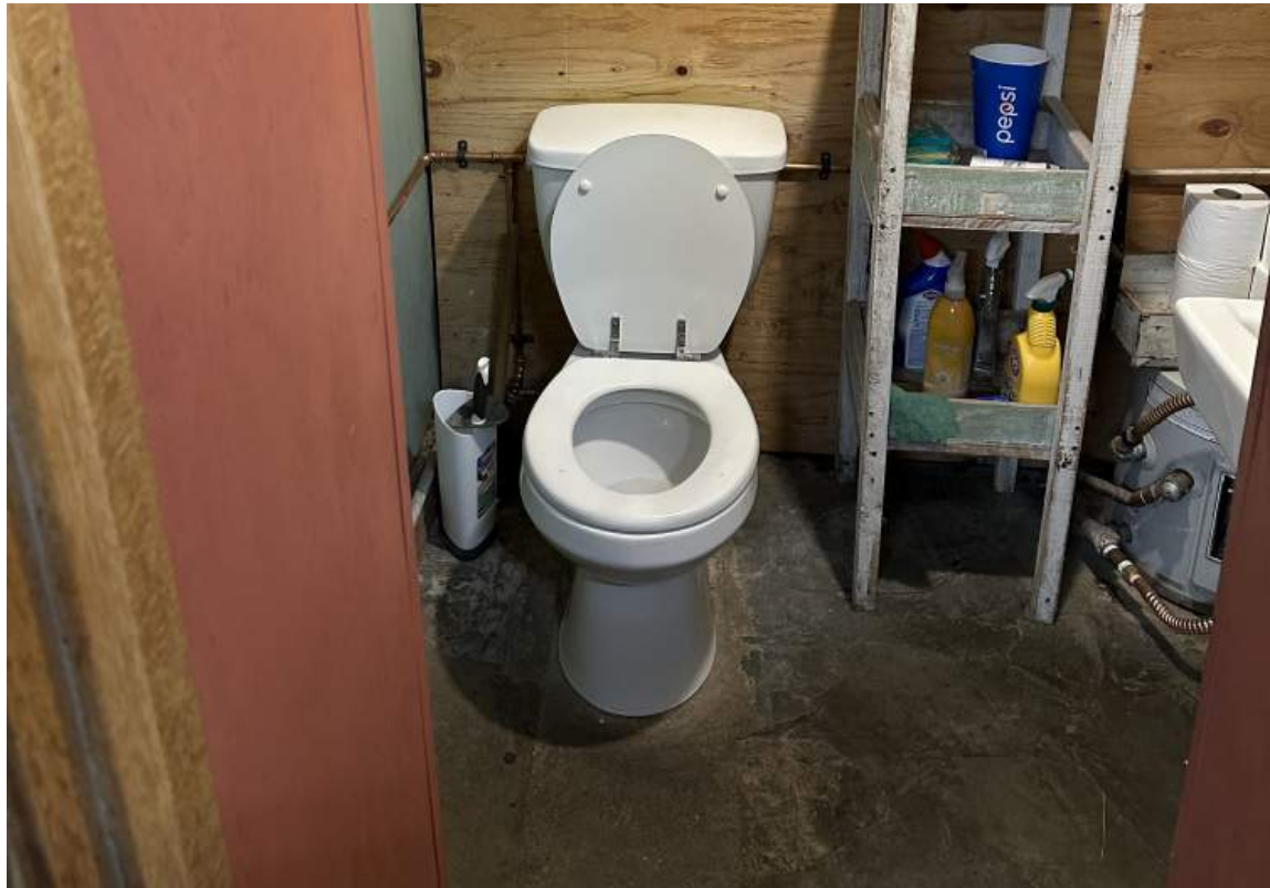
VIEW OF THE TOILET AT THE REDLAND STORE, WHERE GREEN DYE WAS INSERTED. GREEN DYE WAS IMMEDIATELY OBSERVED IN THE FORMER UIC, AND IN THE ON-SITE CATCH BASIN SHORTLY THEREAFTER.
