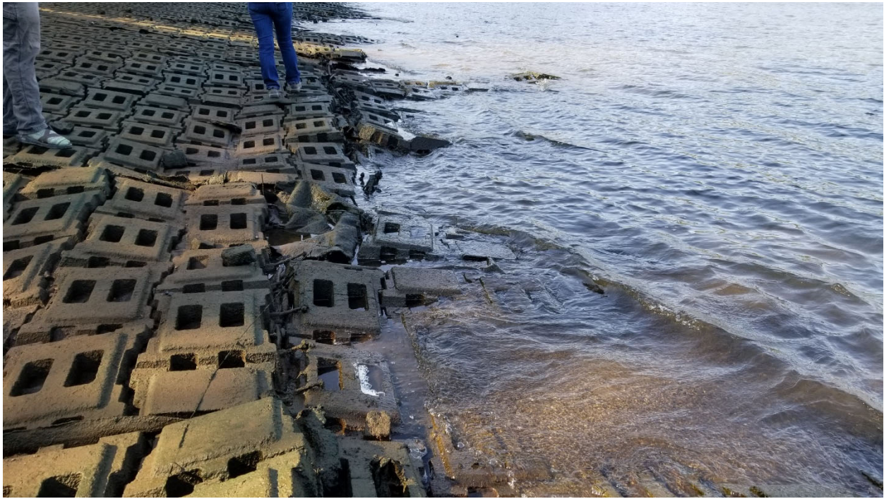
Photograph 4: Buckled ACB along center portion of ACB in Willamette Cove. View facing southwest.
