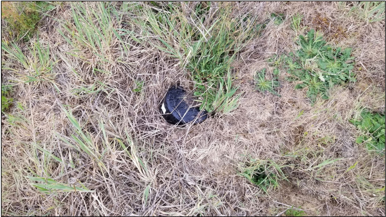
Photograph 5: PVC riser and cap protruding through the soil cap and presumed to be a storm sewer cleanout.
