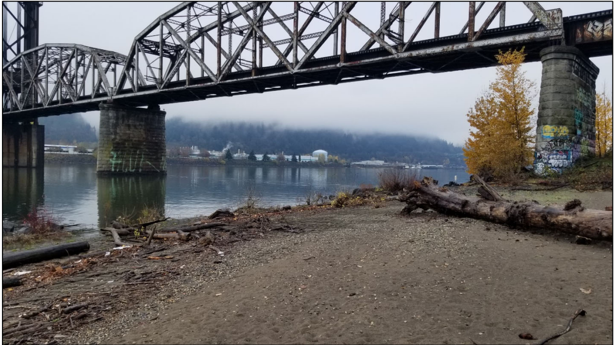
Photograph 1: High tide water levels along the Willamette River shoreline. View facing northwest.
