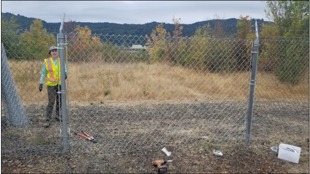
Photograph A13: Replacement of fence fabric section where hole was cut into western perimeter fence. View facing southwest (August 2021).
