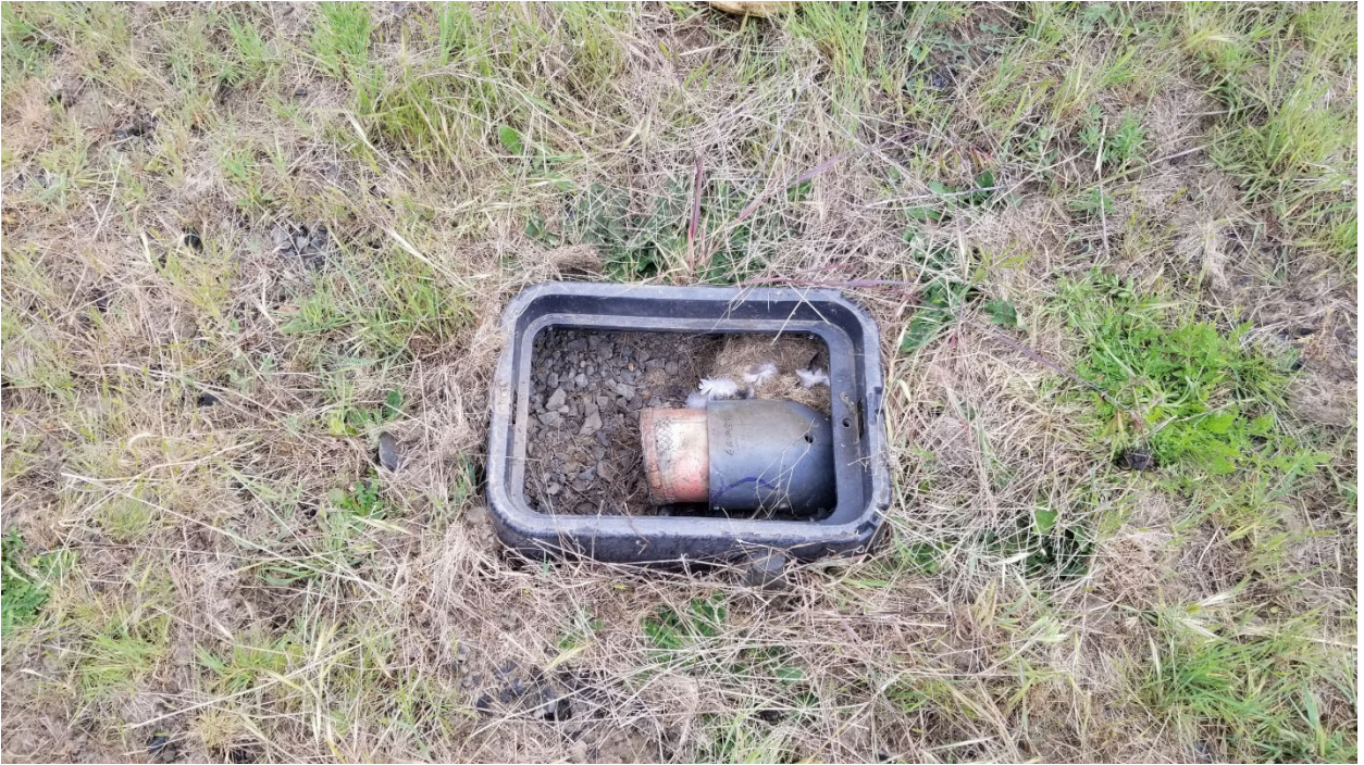
Photograph 6: Rodent nesting inside the gas vent vault box at GV-3.
