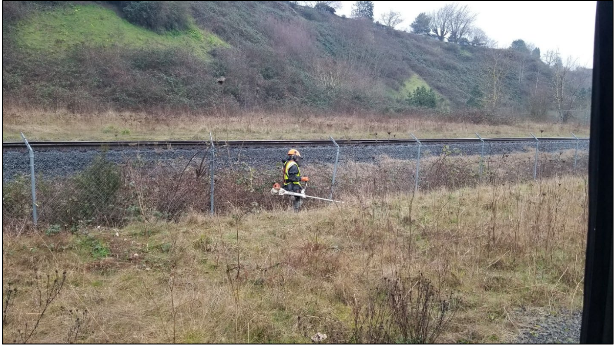
Photograph A7: Weed whacking and removal of blackberry vines growing over eastern perimeter fence. View facing southeast (March 2021).
