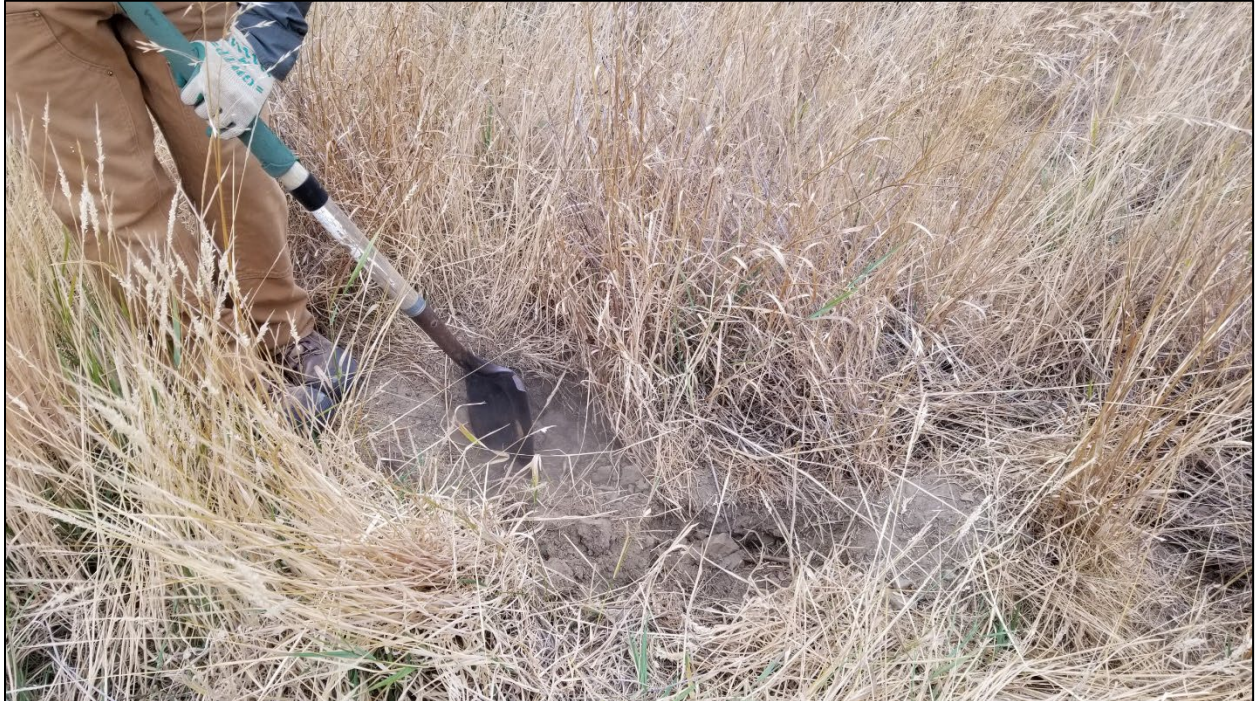
Photograph A12: Collapsing animal burrows in the soil cap and filling in with aggregate base rock material. Burrows were located in the vicinity of MW-48s (August 2021).
