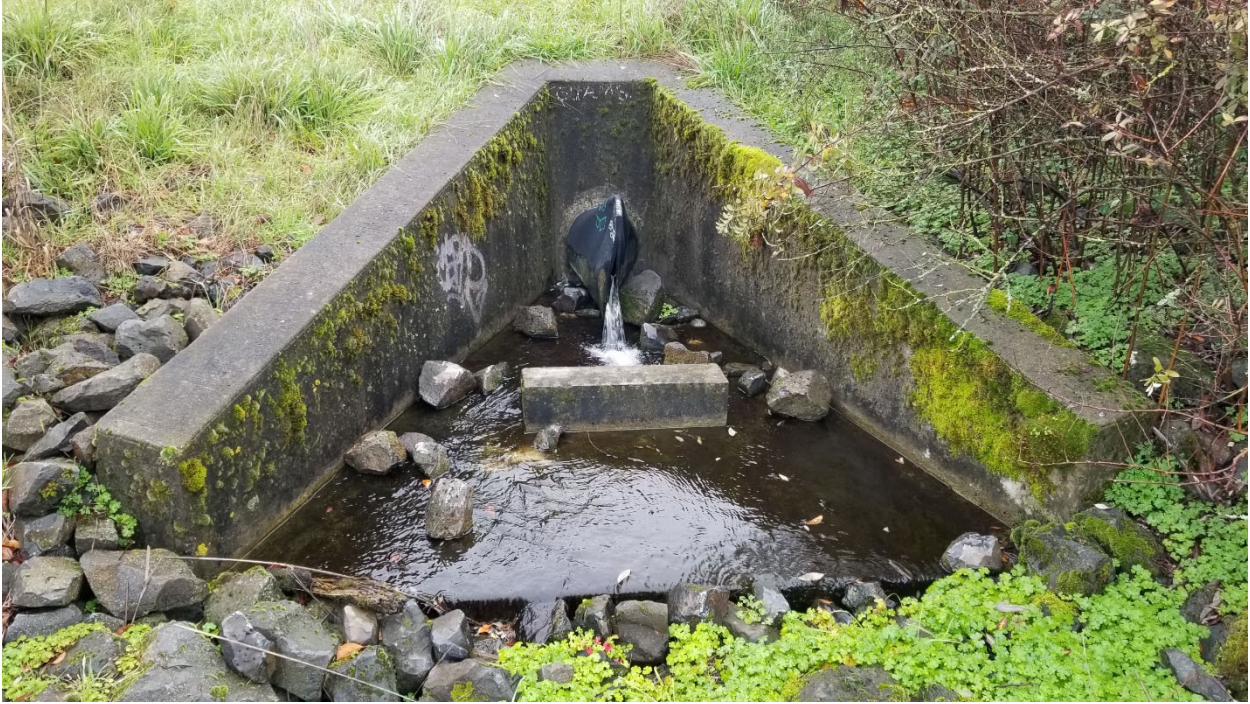
Photograph 3: Stormwater discharge through outfall. Estimated flow rate of 10 gallons per minute.
