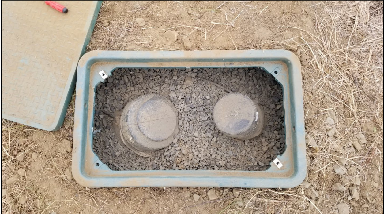
Photograph A10: Installation of vault box for stormwater conveyance piping cleanout CL-4 that was previously buried in the soil cap (August 2021).
