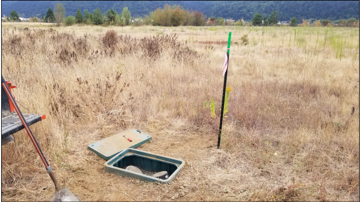
Photograph A11: Installation of marked T-post for location of newly installed stormwater conveyance piping cleanout vault box at CL-4. View facing southwest (August 2021).
