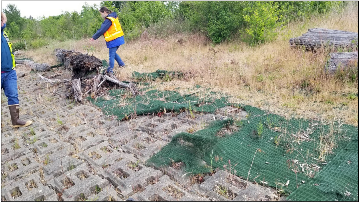
Photograph 3: Loose or torn section of TRM that requires repairs. View facing north.
