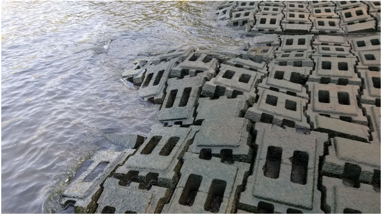
Photograph 3: A second section of buckled ACB from the northeastern end of ACB along shoreline in Willamette Cove. View facing northeast.
