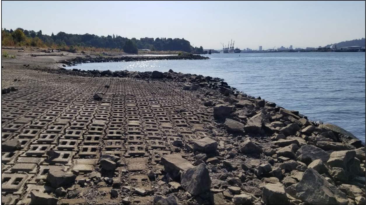
Photograph A15: Low river level conditions showing edge of ACB armoring and transition to rip rap armoring on the sediment cap. View facing southeast (September 2021).
