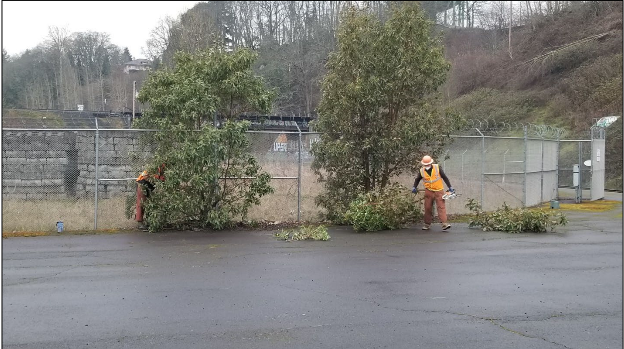
Photograph A6: Removal of trees growing under fence line in paved storage area. View facing north (March 2021).
