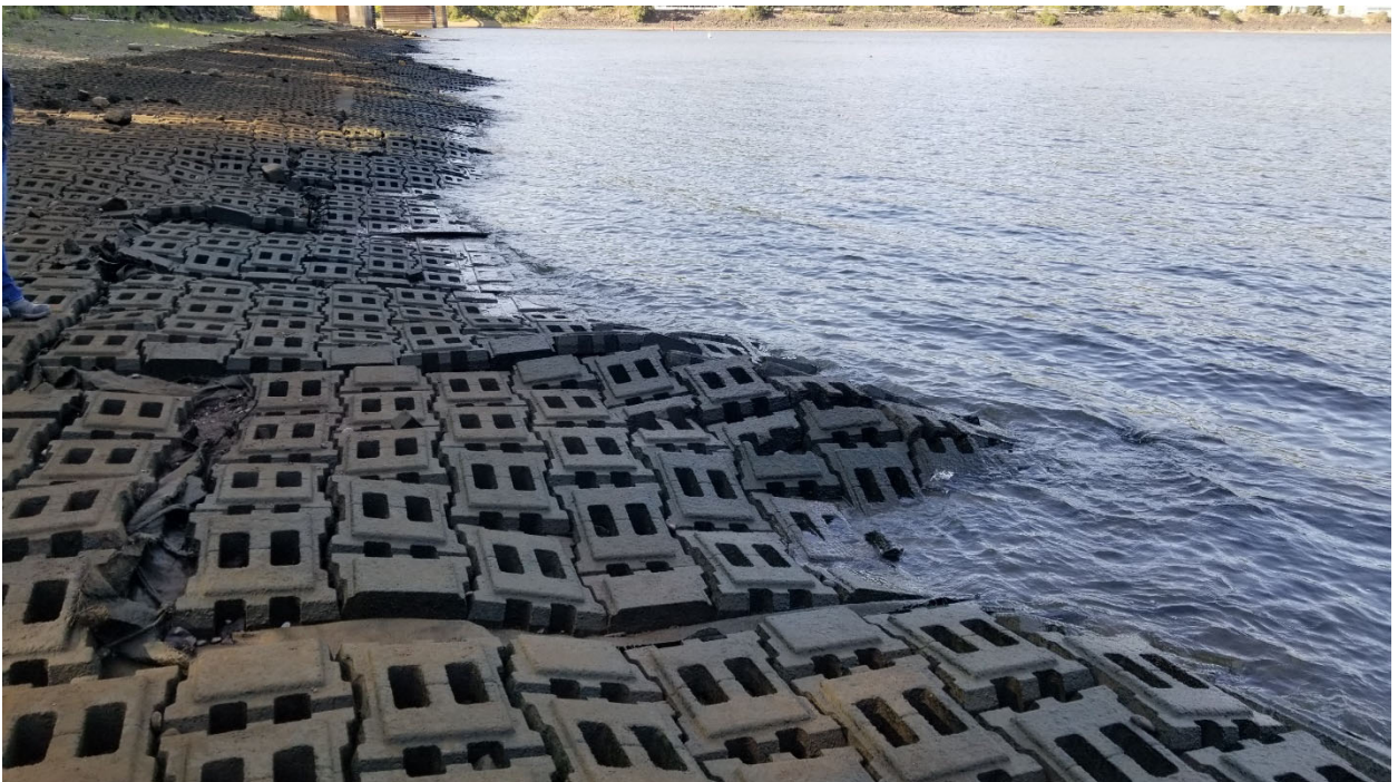
Photograph 2: Buckled ACB from the northeastern end of ACB along shoreline in Willamette Cove. View facing southwest.
