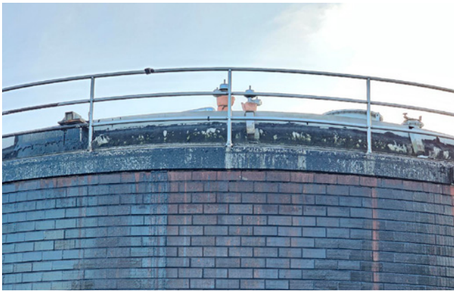
Initial appearance of digester lid
