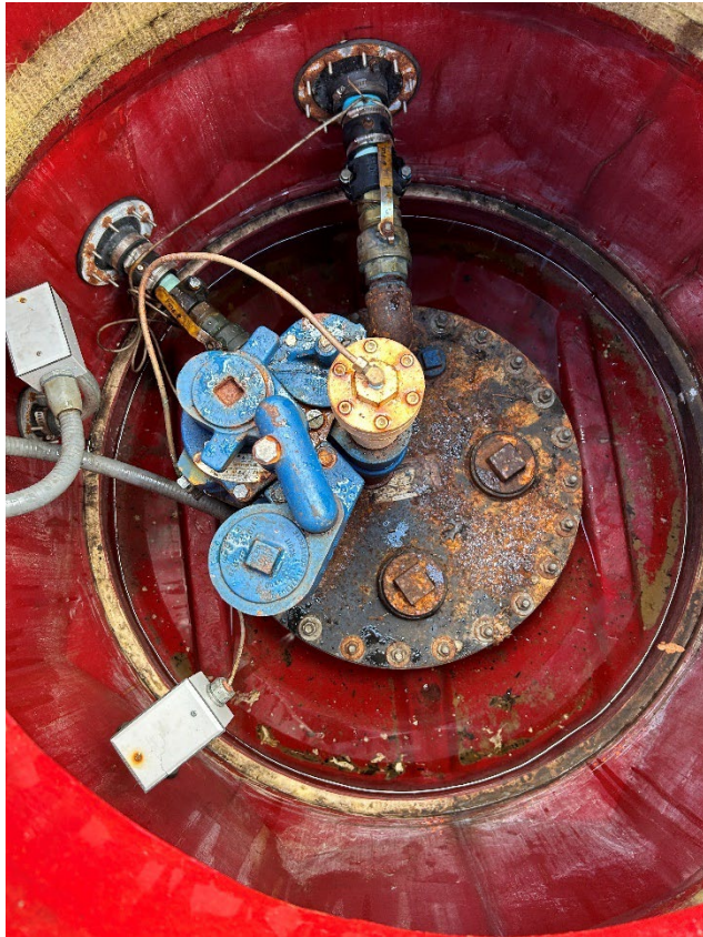
9: Main sump with turbine
