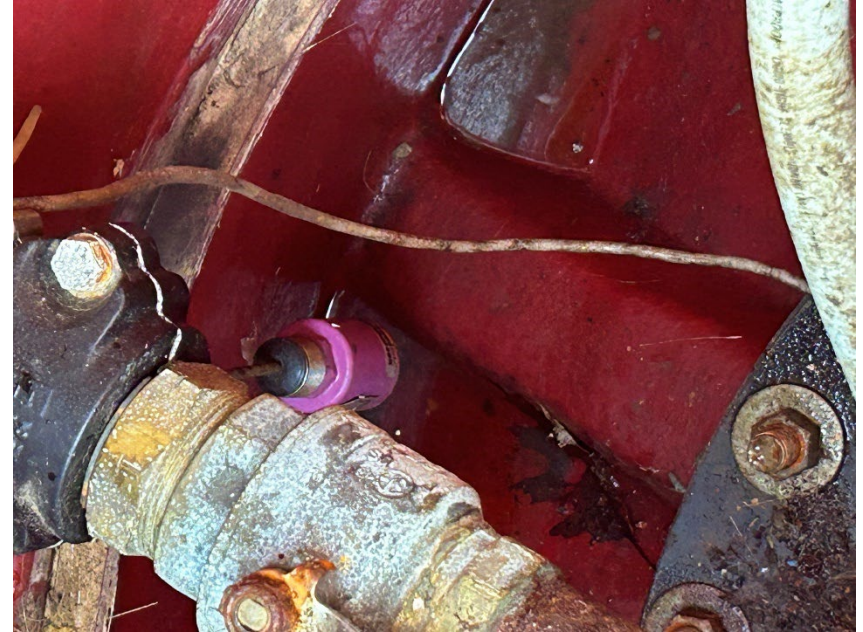
8: Sensor in transition sump
