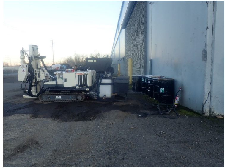
Soil cuttings and decontamination water stored in drums in northwest area of site, pending offsite disposal.
