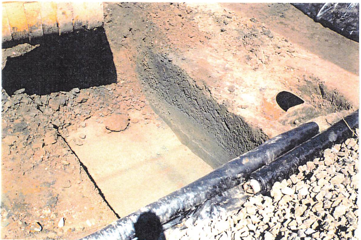
UST DECOMMISSIONING & REMOVAL OF CONTAMINATED SOIL AFTER REMOVAL OF SOUTH UST (NORTH UST VISIBLE IN EXCAVATION)
