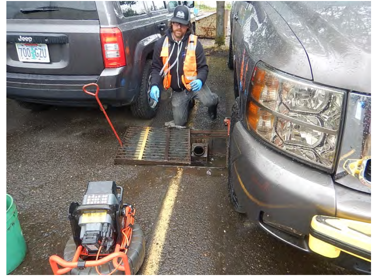
Grate removed from a catch basin prior to being assessed.
