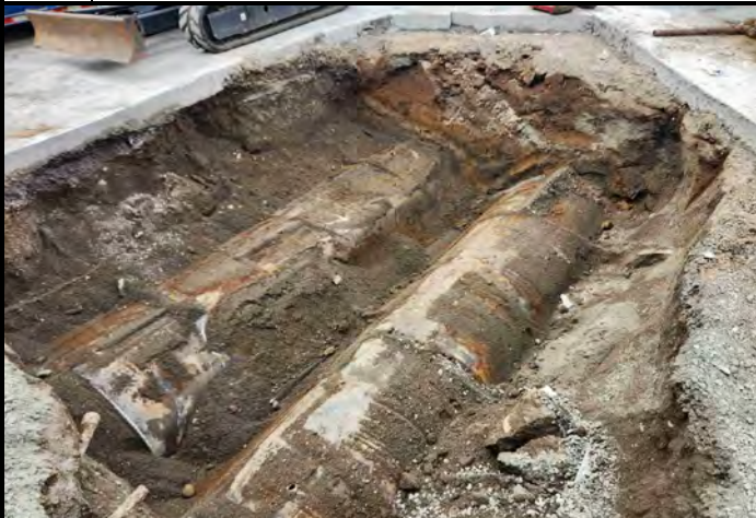
Photo #3: Exposed USTs
