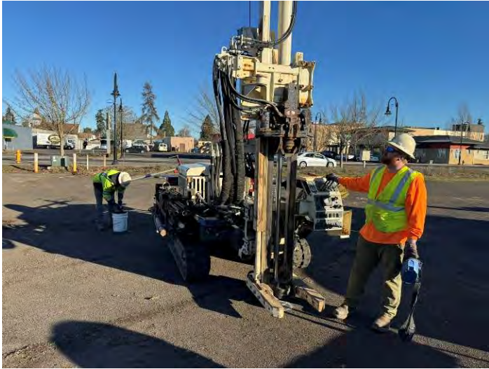
Holt setting up to drill on eastern portion of the site (facing northeast).
