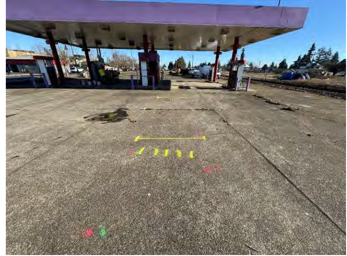
Located product lines extending to canopy/dispenser island (facing east).
