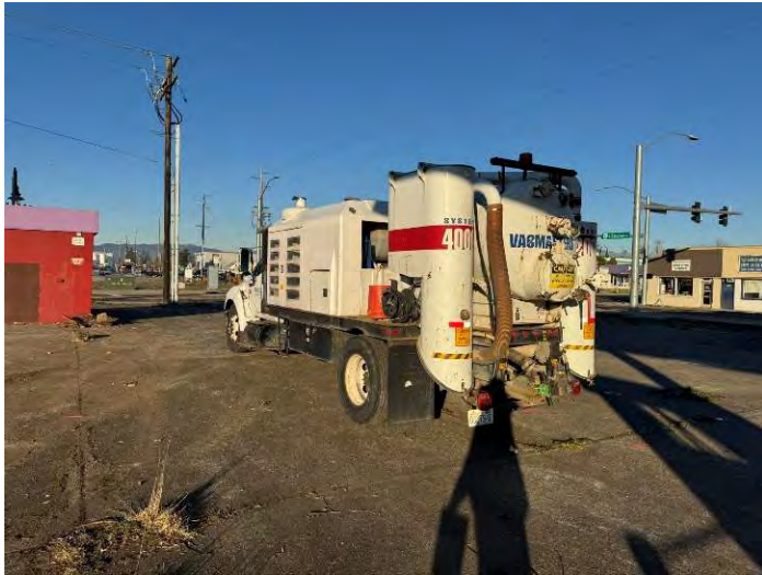
Vacuum excavation truck (Holt) on site to begin clearing boring locations close to utilities/underground disturbances (facing northwest).
