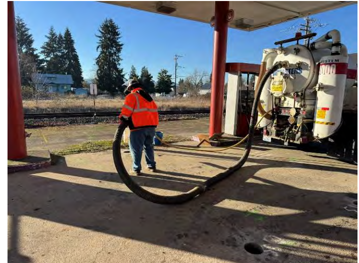
Vacuum excavation truck crew clearing borings under southern portion of canopy (facing south).
