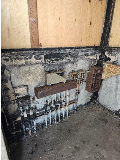
Burnt electrical work to left of kiosk entrance.
