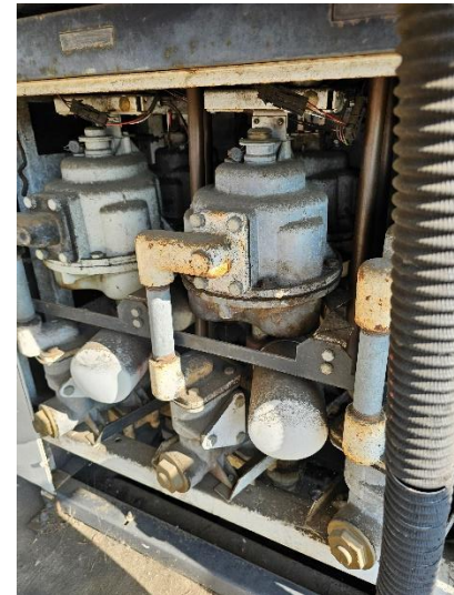
Pump with front cover removed, exposing pump systems inside.
