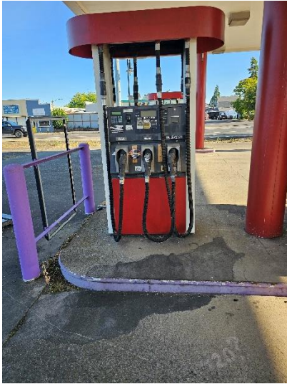
Spill/stain in front of pump on east side of the property.
