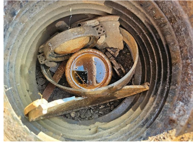
8k Unleaded UST with water in fill pipe.
