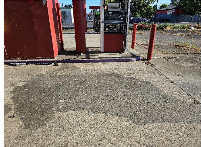
Spill/stain in front of pump on west side of property.
