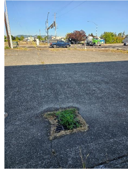
Drain on western side of property (dry, no liquid inside).
