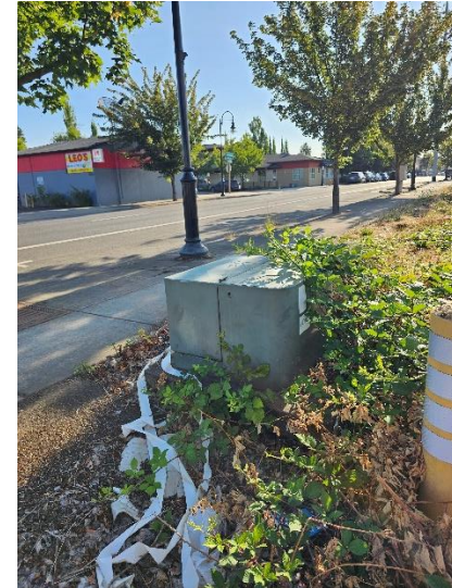
Transformer on northeast corner of property (PCB free).
