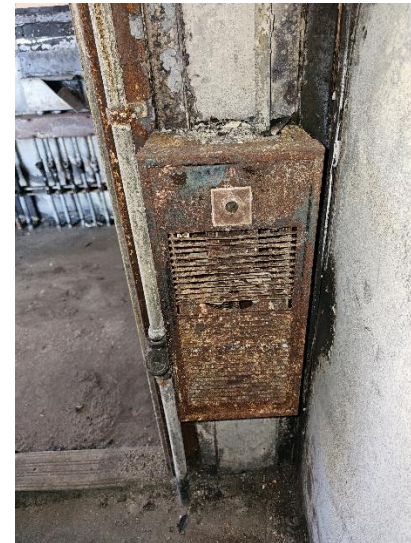
Burnt electric heater in kiosk area.
